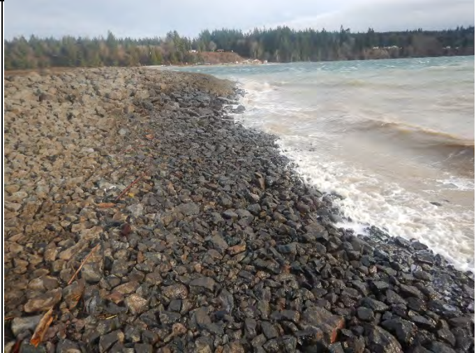
Comment: Erosion Area 3 – west of transload area
