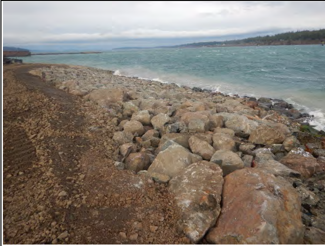
Comment: Erosion Area 1 – north of Eastern Wharf
