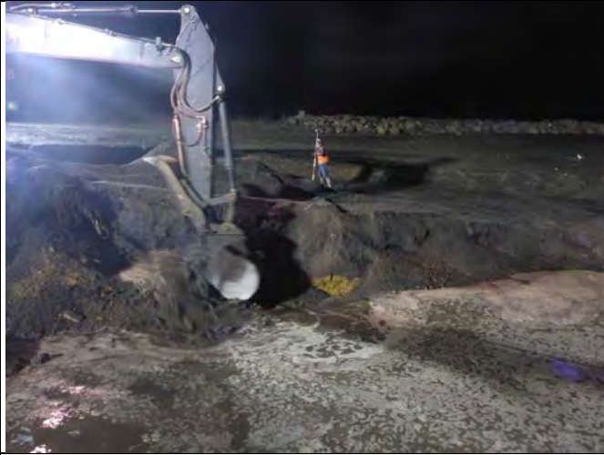
Comment: Over-excavation of wood waste in SMA-1
