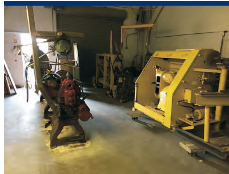
Photo 24 Equipment left in northern portion of Maintenance building near estimated location of four nested USTs.
