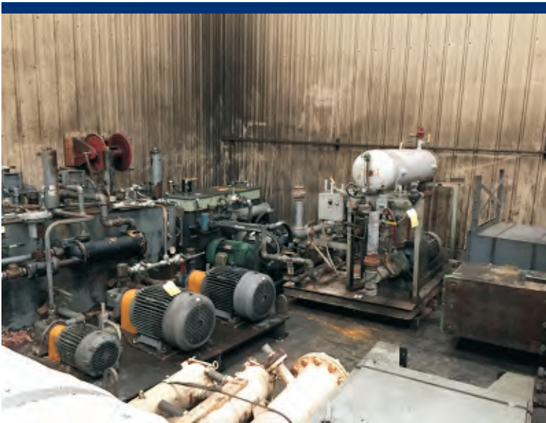
Photo 47 Northwest corner of steam cleaning facility with staining on walls.
