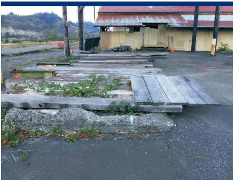
Photo 23 Concrete trench box assumed to be associated with old planer feed line (beneath wood planking).
