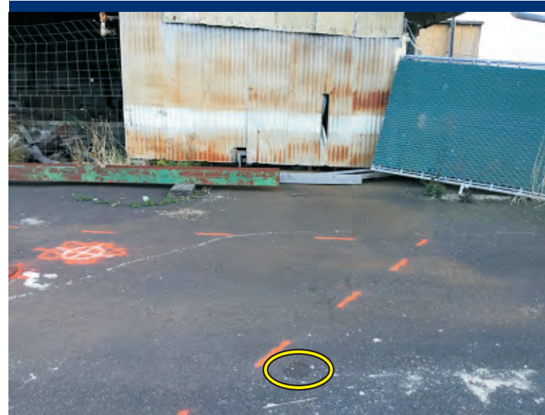
Photo 18 Small asphalt patch assumed to be associated with GP-1.
