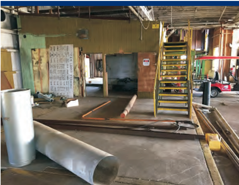
Photo 7 Northern interior of Planer Building. Green walled room may have been old spray room.
