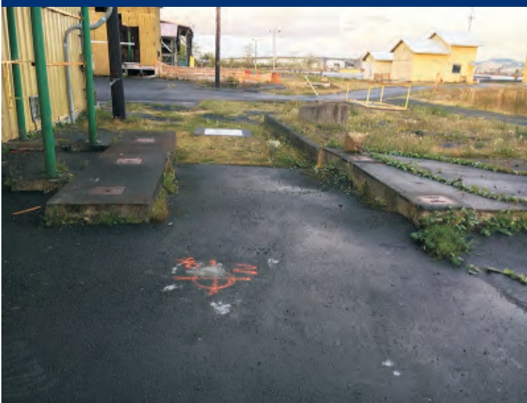
Photo 5 Boring location MS05 and transformer vault.
