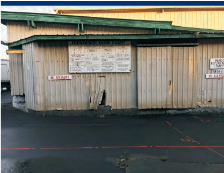
Photo 43 Sign on south side of hazardous material storage shed, showing storage organization and handling decision tree.
