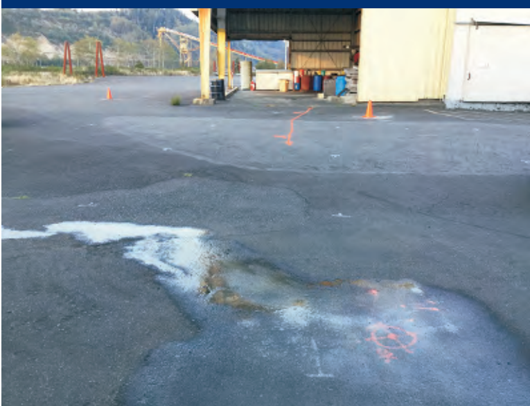
Photo 9 Location MS06, before sampling. Location FC02 in background was where petroleum odors had been noted.
