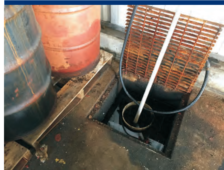
Photo 30 Oil remaining within blind sump in fuel and chemical storage building.
