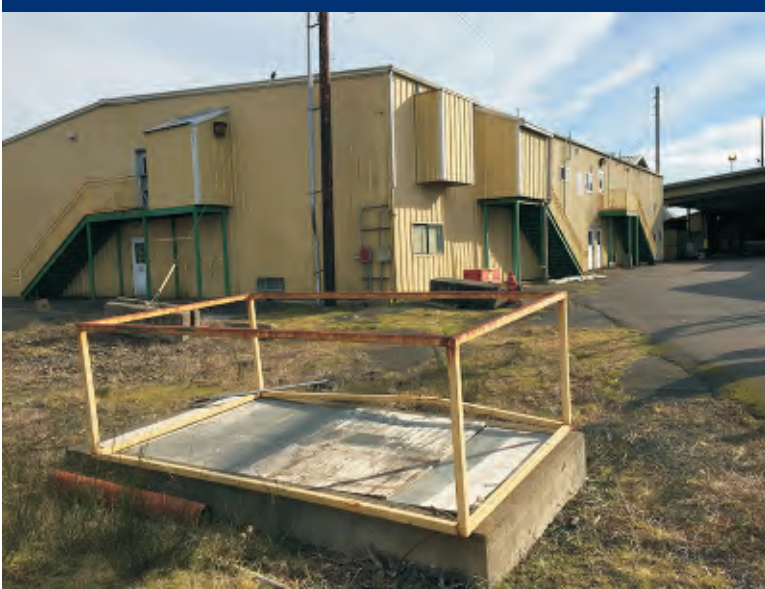
Photo 5 Fire suppression system vault and west side of maintenance building.
