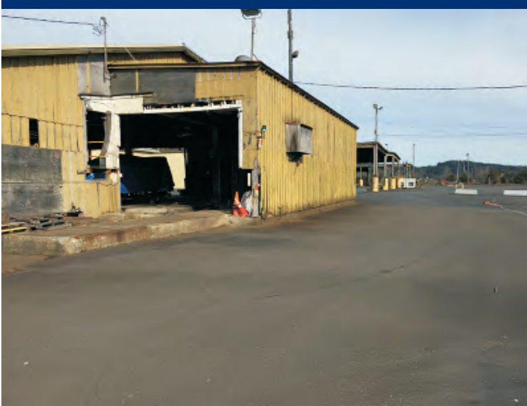
Photo 21 South side of planer bldg where paint waste UST release was reported.
