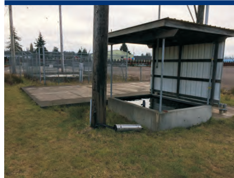
Photo 42 Containment interpreted as location of backup generator diesel AST. Former transformer pad behind.
