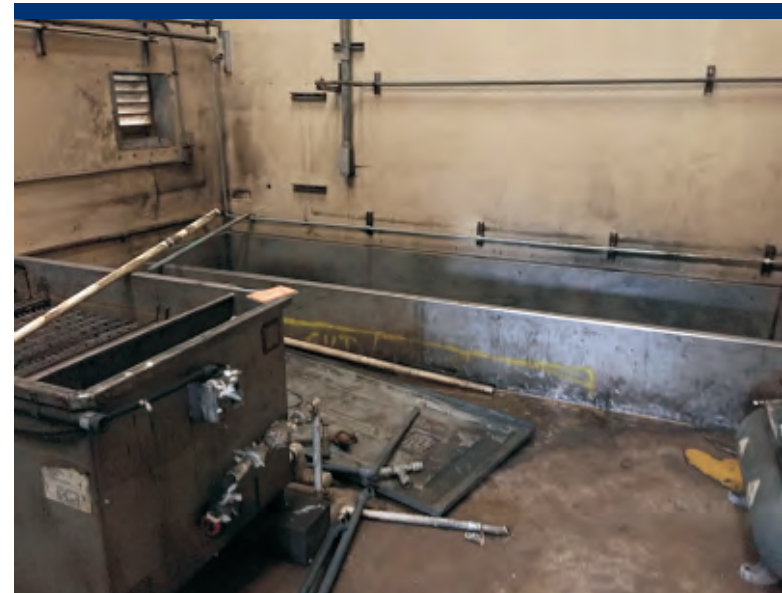
Photo 48 Steel basins in water treatment system room.
