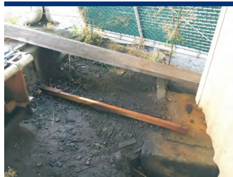
Photo 24 Stained soil at west wall of planer building, where conveyor feed appears to have entered building.
