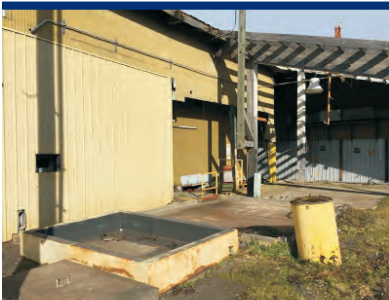
Photo 11 Pads and containment curb on south side of Planer Building. Former use of both unclear.
