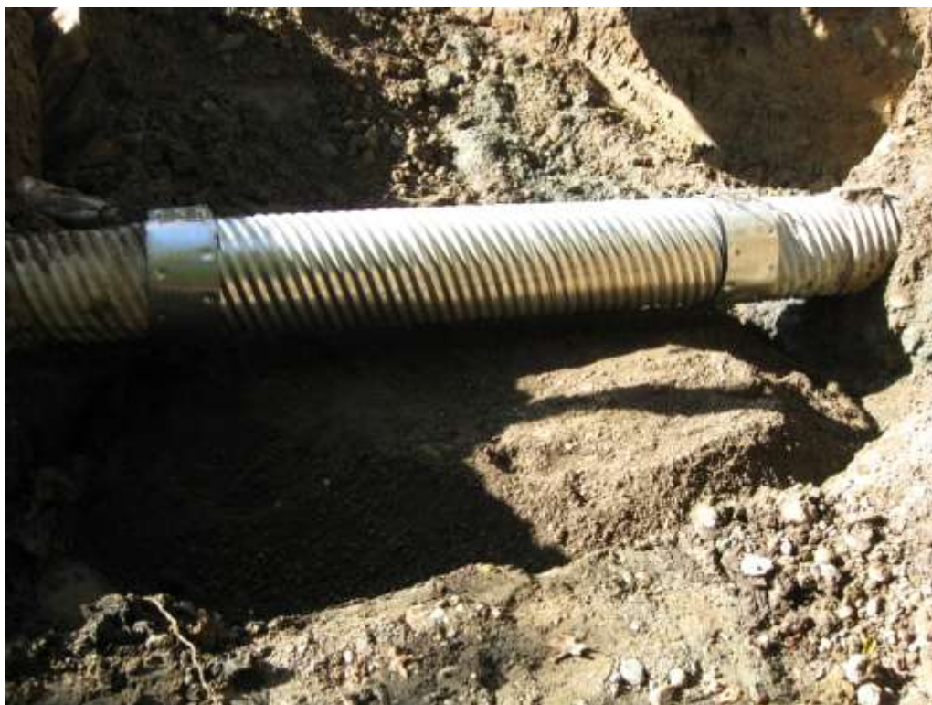
Photograph 16: New section of culvert with banding on north portion of Site by 218 th Street, October 19, 2010.
