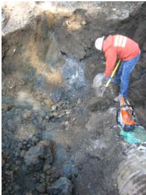
Photograph 15: Removing slag and lime ash around culvert on north portion of Site, October 19, 2010.
