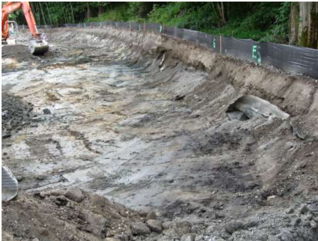
Photograph 9: Clean silt, clay bottom, and old liner with pea gravel on east portion of Site, September 7, 2010.
