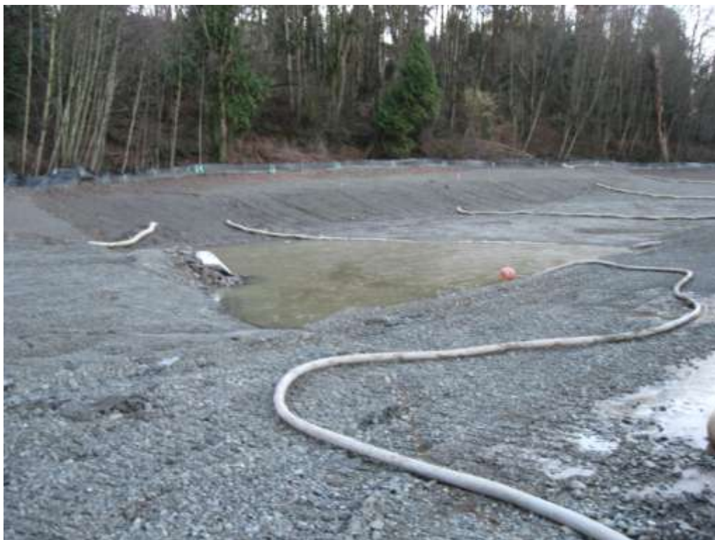
Photograph 20: Erosion control wattles, ponded water, and new culvert on east half of Site, February 1, 2011.
