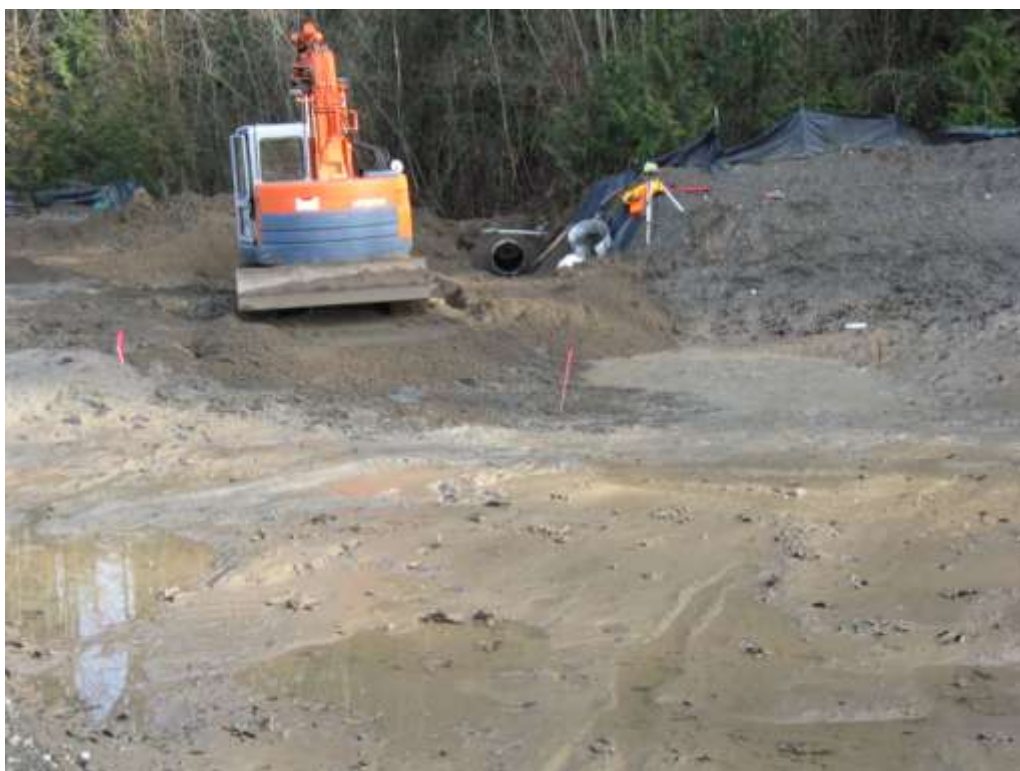
Photograph 18: Trench excavation between ponded water and detention pond to install new culvert, January 26, 2011.
