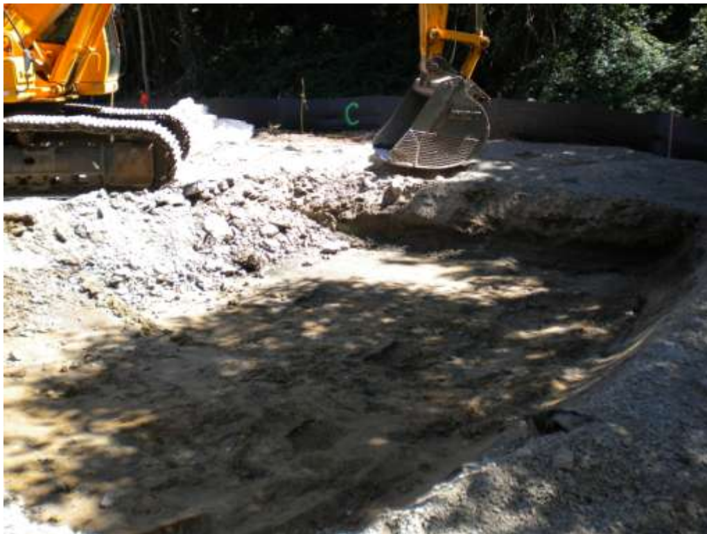
Photograph 5: Removing slag on south portion of Site to install wheel wash, August 22, 2010
