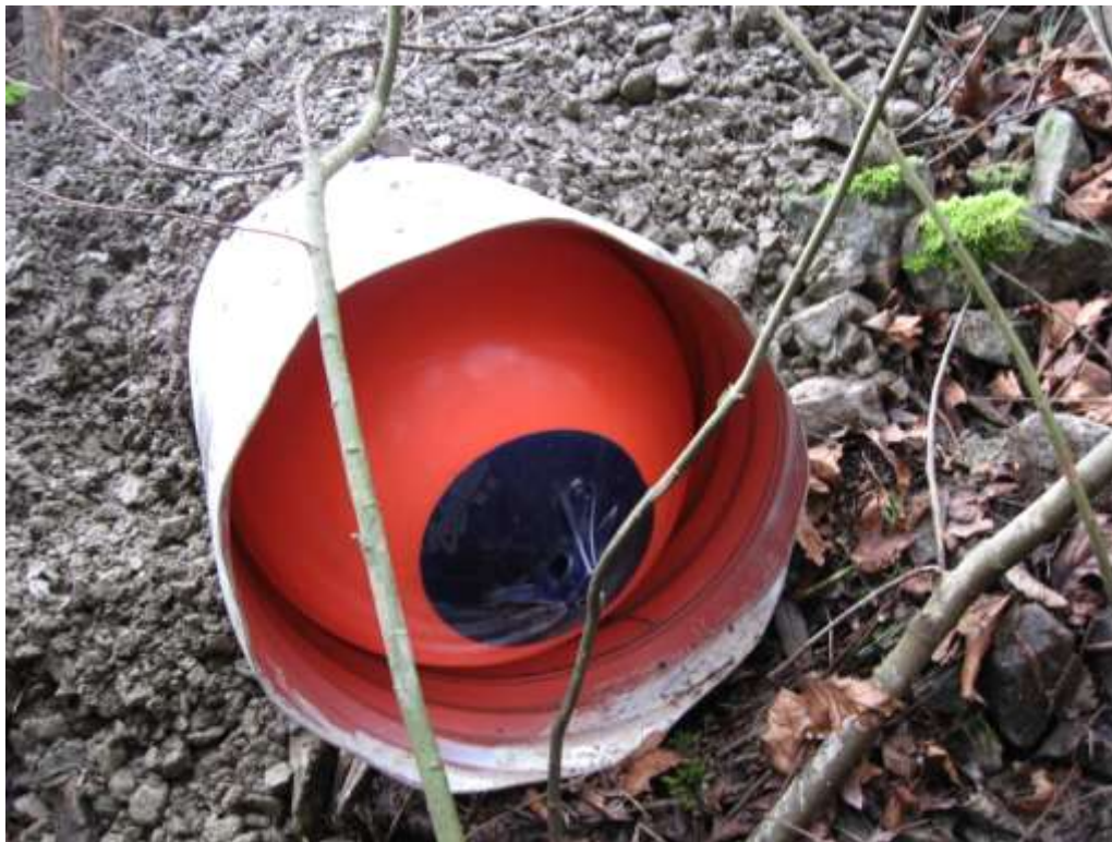
Photograph 19: Rubber buoy in outlet of new culvert on north portion of Site before turbidity test, January 27, 2011.
