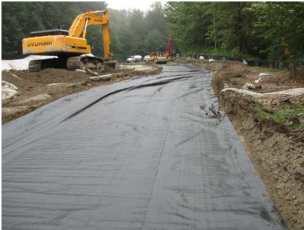
Photograph 13: Laying down Geotech fabric to construct new haul road on west side of Site, September 22, 2010.
