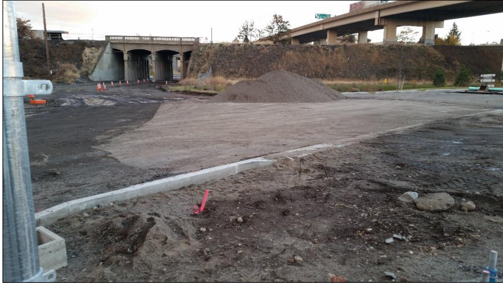
3. View of City of Spokane improvements, at east Site boundary, where MLK Jr Way intersects North Erie Street (looking south).
