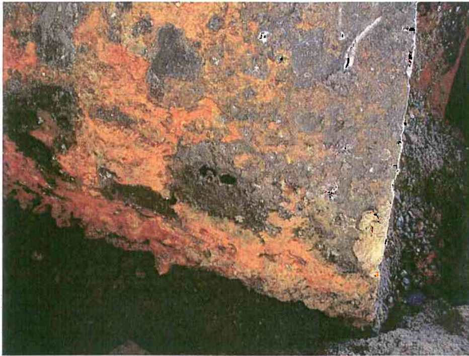
Typical holes and rust observed on underground storage tank. (April 11, 2008)
