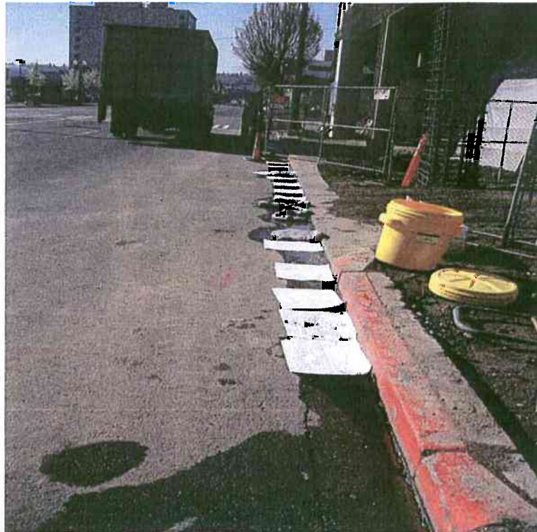
Cleanup action for petroleum spill on asphalt during removal looking south. (April 11, 2008)
