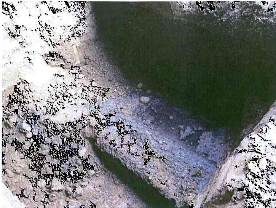
Example of blue-gray soils eastern portion of excavation (approximately 8.5 feet bgs). (April 14, 2008)
