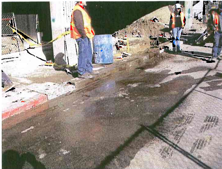
Petroleum spill on the asphalt from removal. (April 11, 2008)
