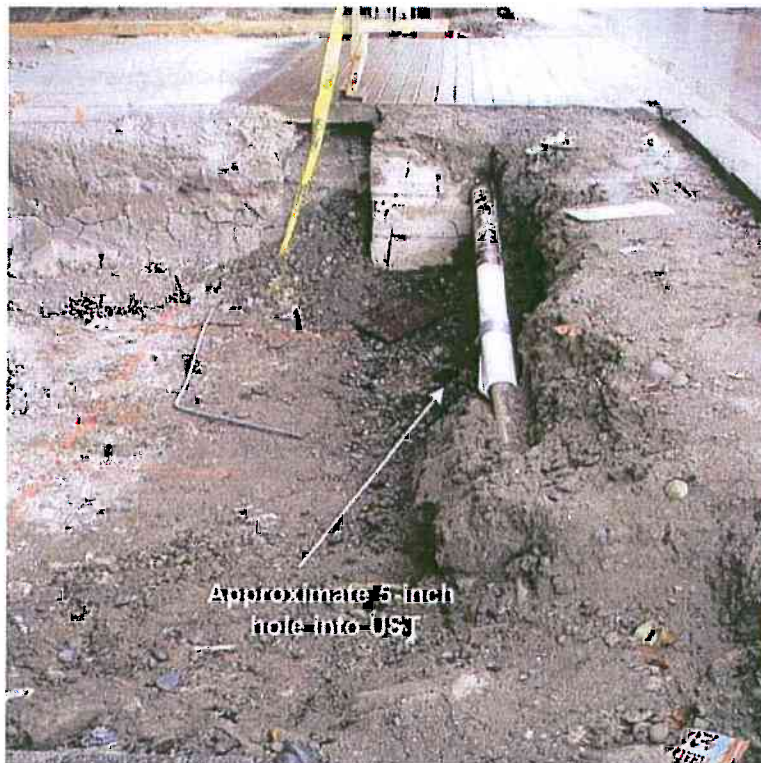
Discovery of UST looking north. Orange paint shows the location of the new footing. Gray pipe shows the approximate southwest corner of the UST. White pipe is an abandoned phone line. (April 4, 2008)
