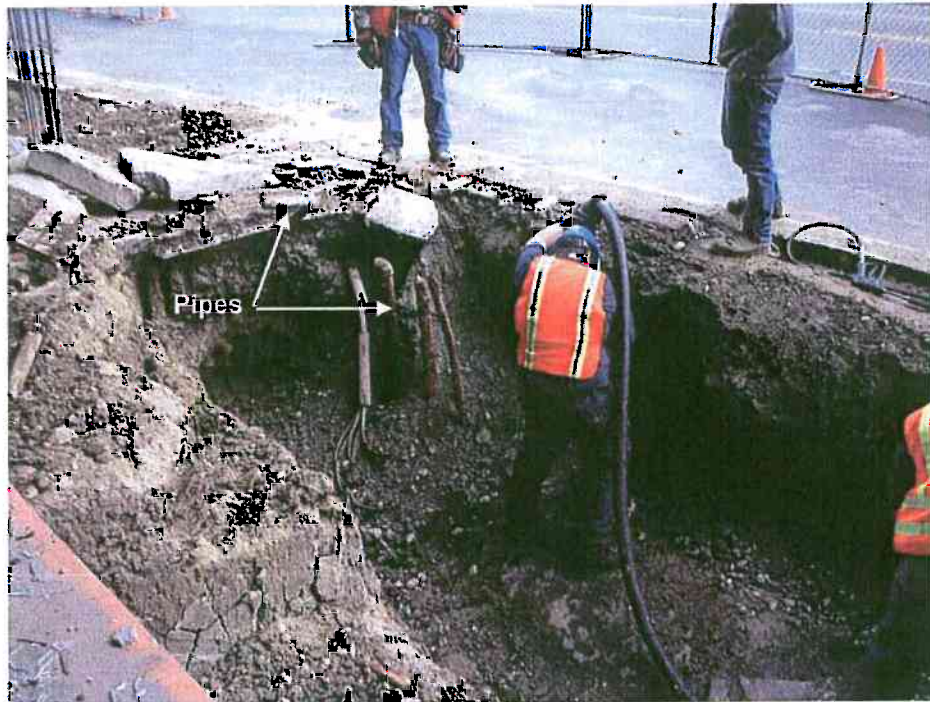
Phoenix Environmental removing oil and sludge from underground storage tank (UST) looking northeast. (April 10, 2008)
