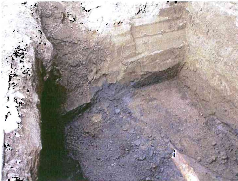
Final extent of excavation on south wall. South wall soil sample (Conf-S.Wall) collected in blue-gray soils (April 14, 2008)
