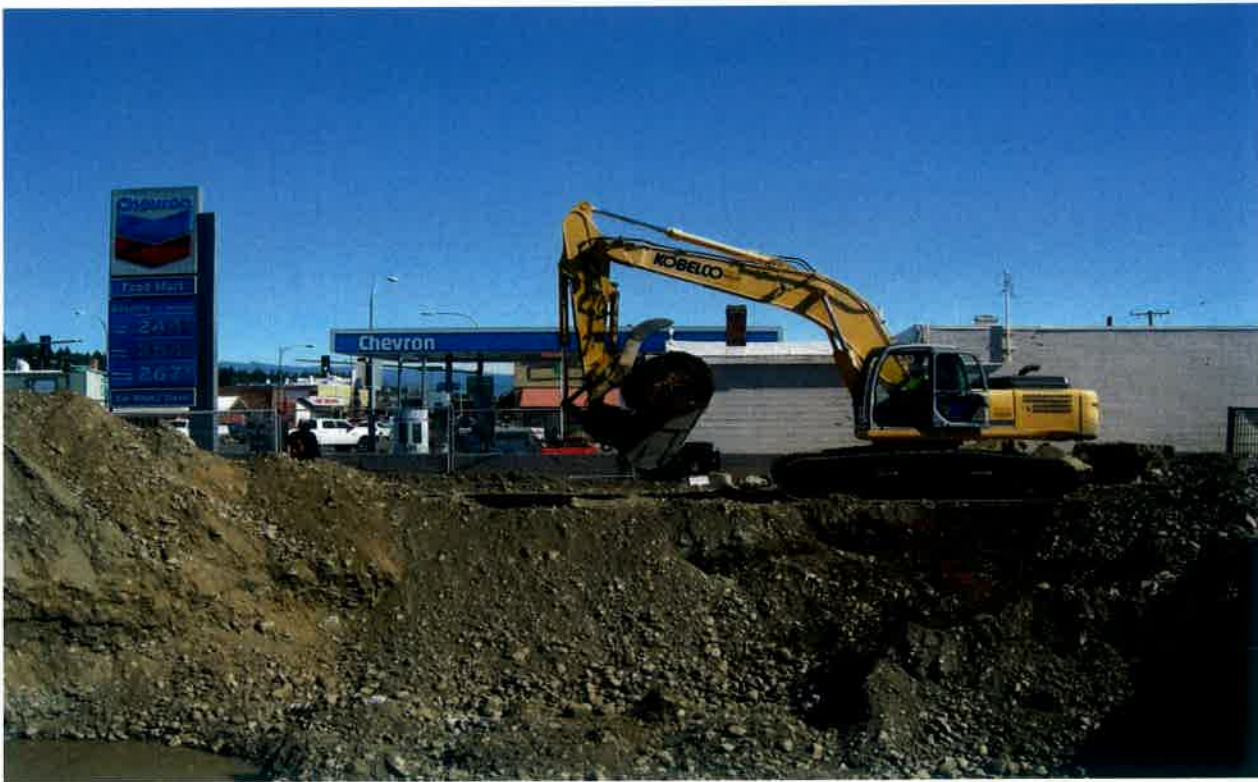
Mr. Wilkerson directs the excavator Operator to remove the "Surprise Tank" for transportation.
