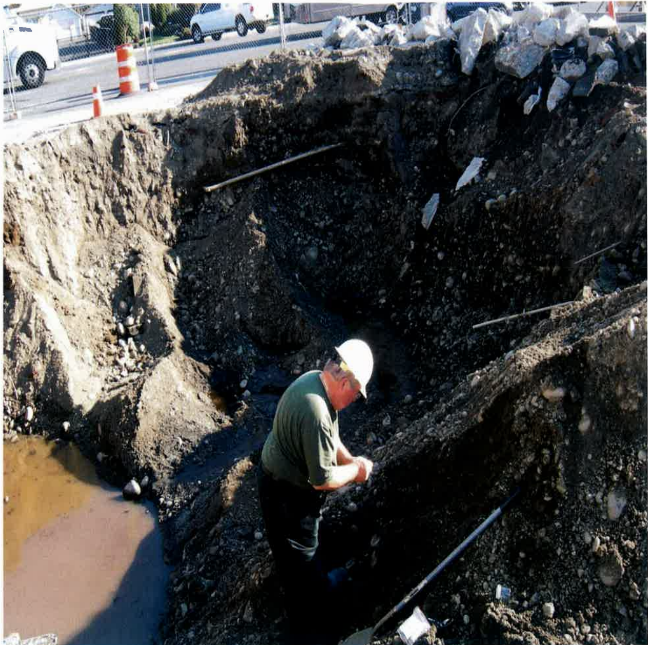
Webster investigated the soils remaining in the Tank Pit Nest after the removal of the five USTs. (Note the number of small pipes protruding from the east bank of the pit wall.)
