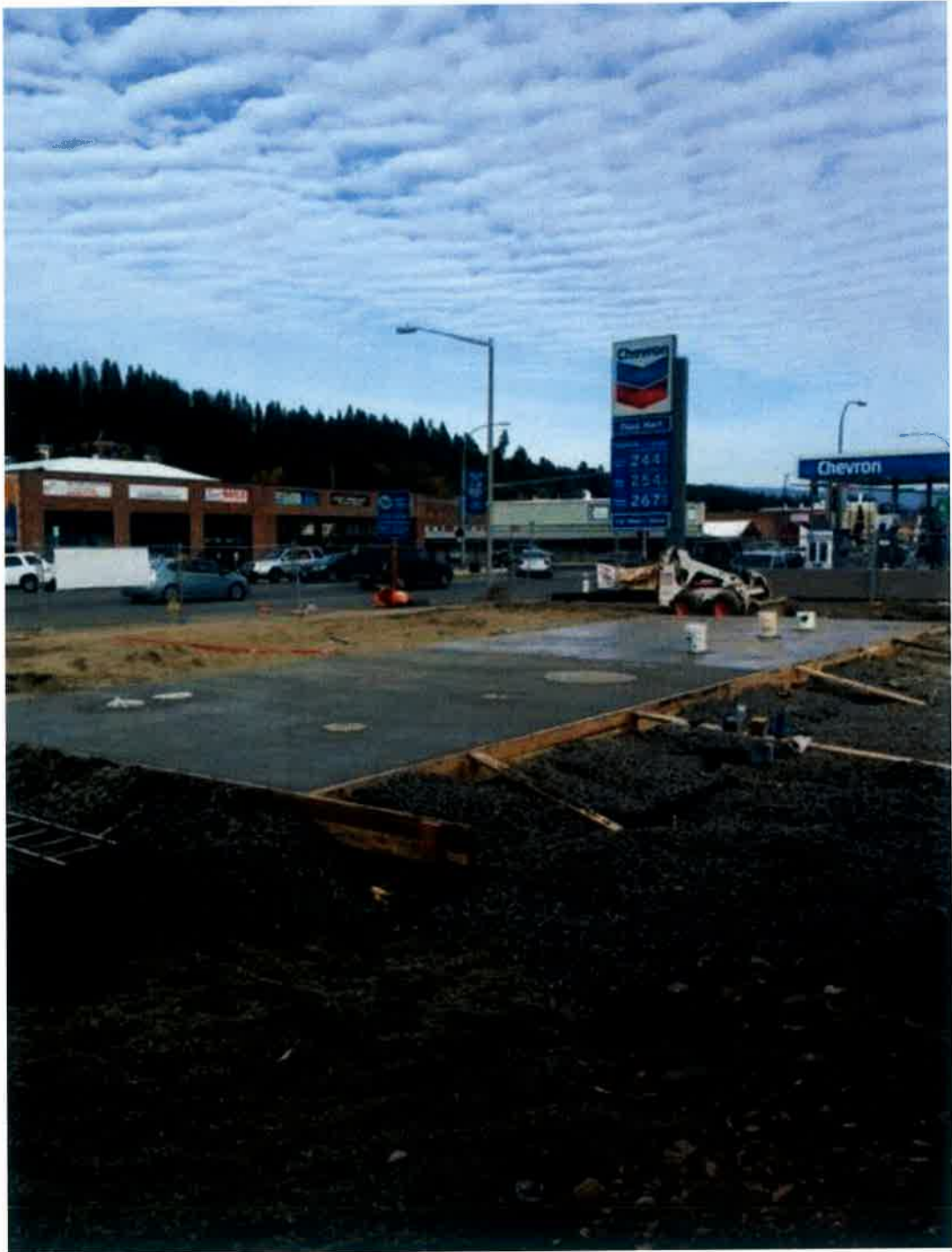
A “Concrete Slab” was poured atop the Tank Pit of the two new USTs
