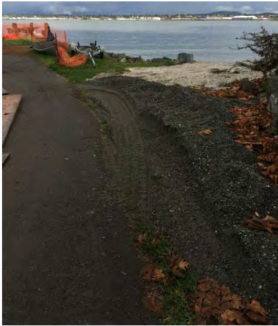
Crushed gravel that shall be removed before project completion
