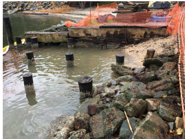
Removed Wharf and shoreline condition underneath. Contractor directed to remove wood debris before boom is removed.
