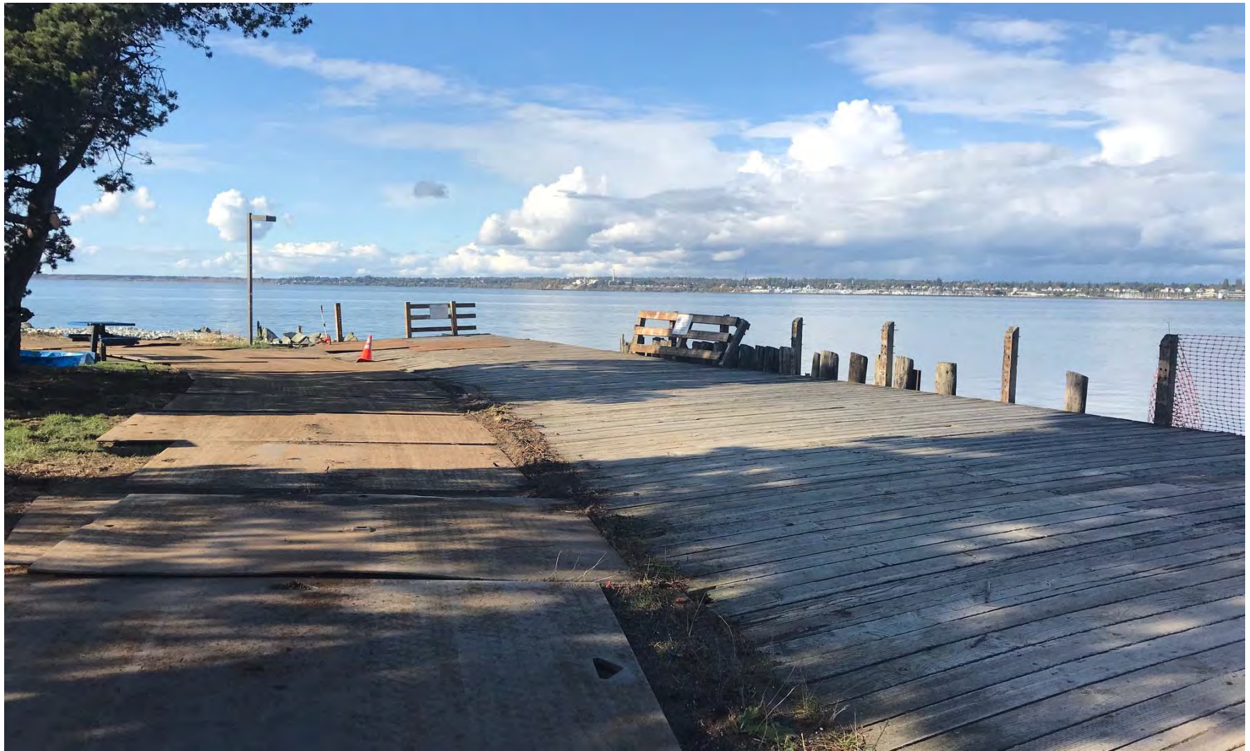
1. Wharf deck conditions; 3:30pm. Piles stored on the deck have been removed. Decking still in-place.
