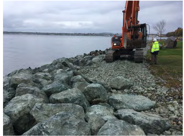
Armor stone placement, not approved as pictured, some additional movement was needed.
