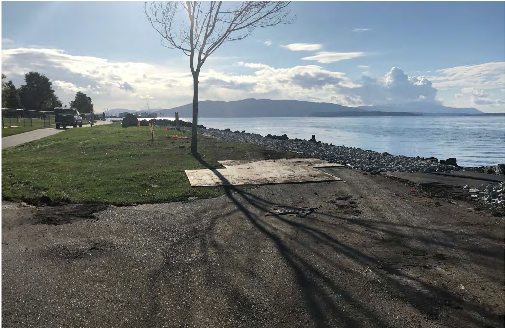
1. Riprap bedding placement along shoreline to provide stable and flatter surface for boulder placement. Geotextile visible at right.
