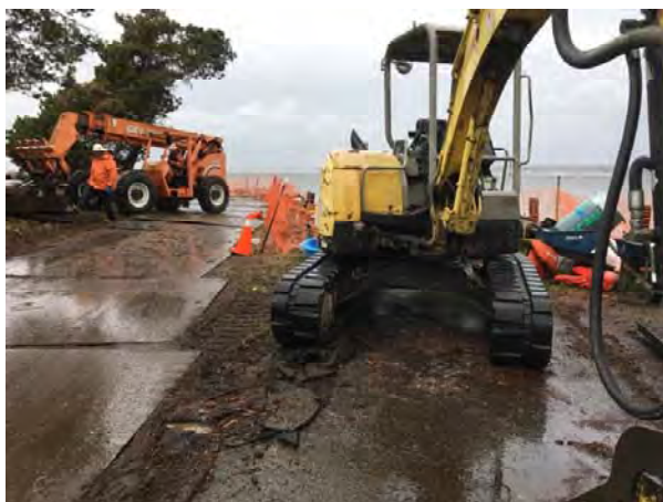
Pavement damage near wharf
