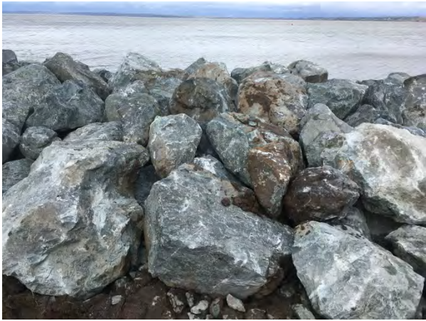
Small, unacceptable rocks atop. Instructed contractor to remove
