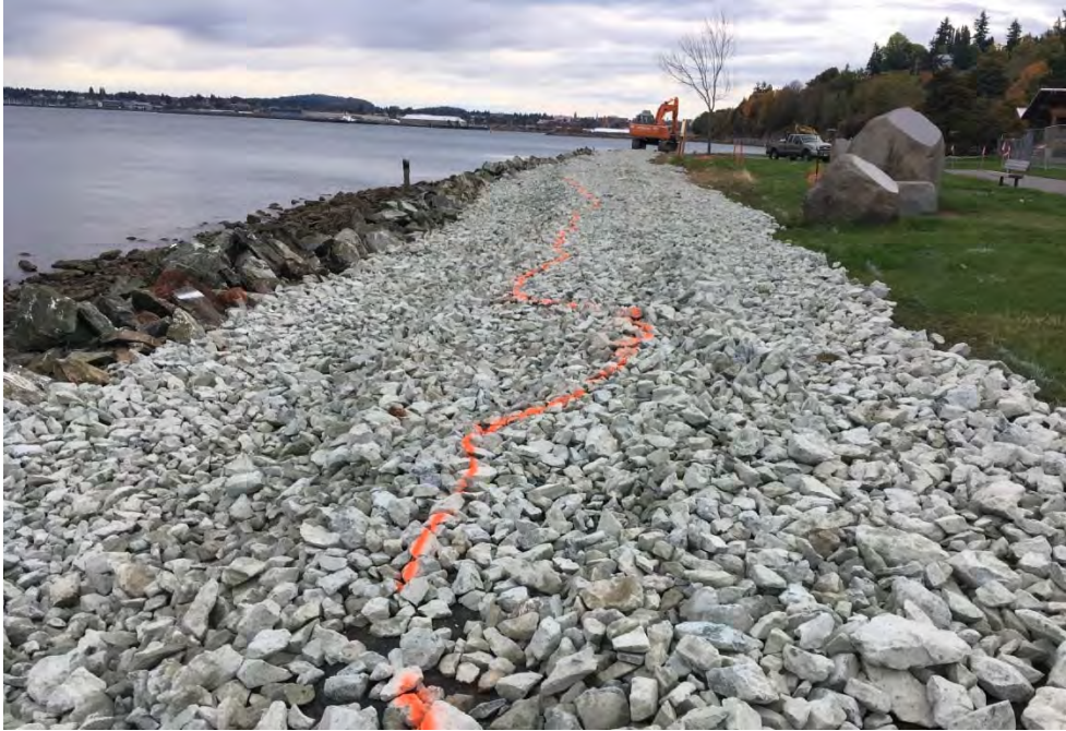
Figure 2. Ground photo showing approved quarry spall placement looking north on the west shore of Boulevard Park.
