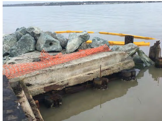
Concrete apron. Contractor asked for direction of how to tie into armor stone berm. Photographed from the west
