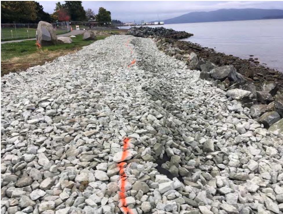
Figure 3. Ground photo showing approved quarry spall placement looking south on the west shore of Boulevard Park.
