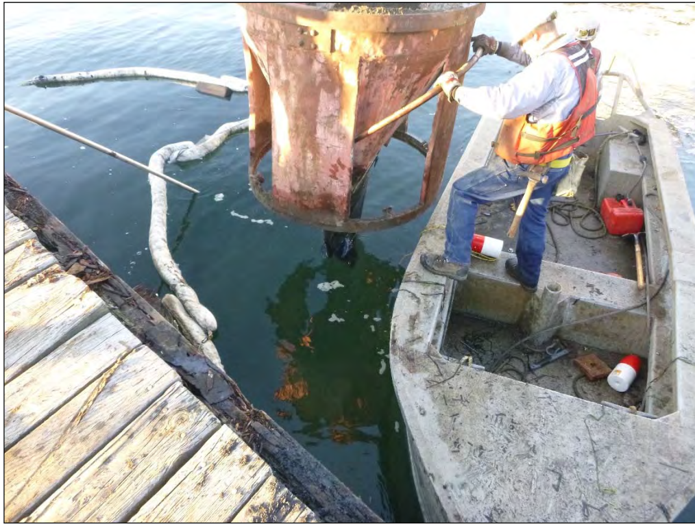
11. Gar-bro bucket filled with sand, ready for drop over previous pile location, located using weight on end of buoy and yellow line placed before pile was pulled.
