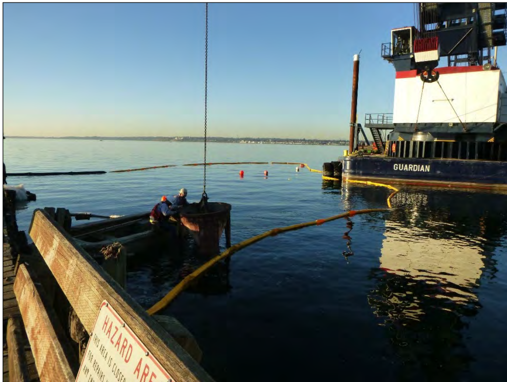
12. Sand drop over previous H-pile location. Other pile locations marked with buoys in background.
