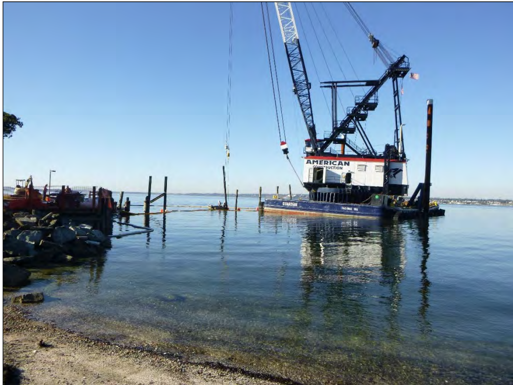
7. Looking northwest at all remaining creosote and H-piles, loosened and ready for extraction.
