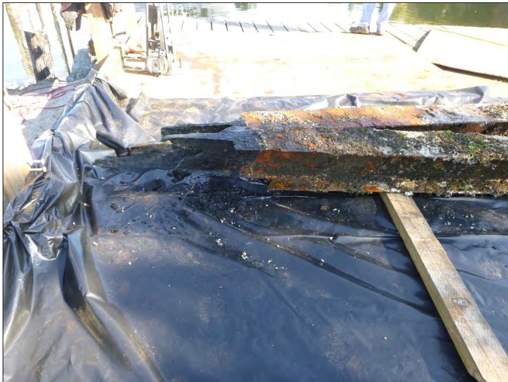
4. Two pulled steel H-piles with substantial rust and corrosion of steel below mudline placed on plastic sheeting for containment.
