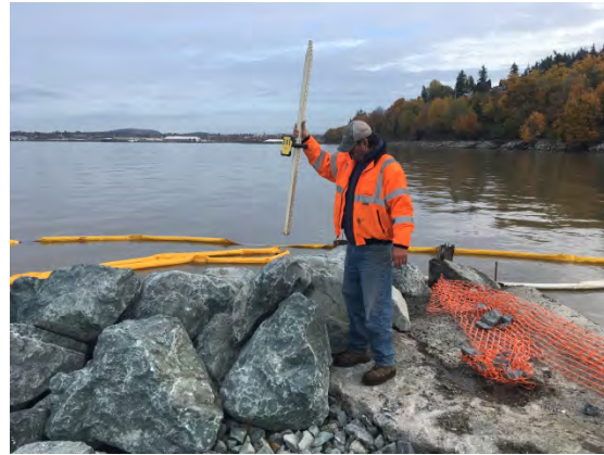
Checking grade, Rick showing 13.5' MLLW. In this location, 13' will be the crest elevation.
