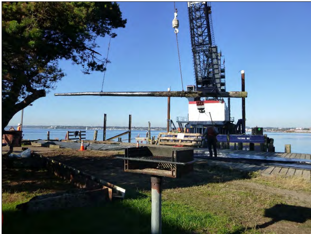
8. Full length of creosote wood pile removed and being placed on plastic sheeting for cutting and loading to disposal.
