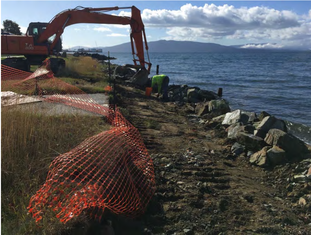
Figure 4. Ground photo showing approved subgrade looking south on the northwest corner of Boulevard Park.
