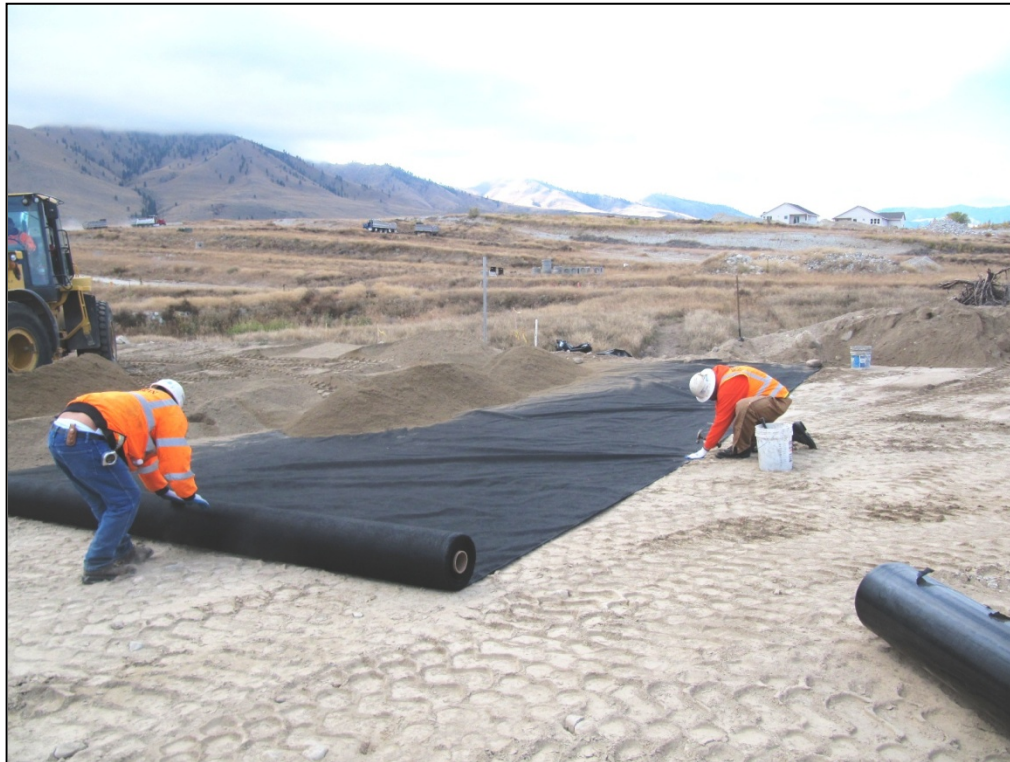
1. Installing the geotextile fabric over contaminated soils in the North Fields area.
