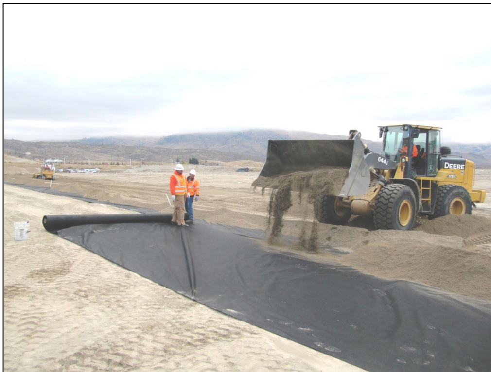
2. Placing the clean fill soil over the geotextile fabric in the North Fields area.
