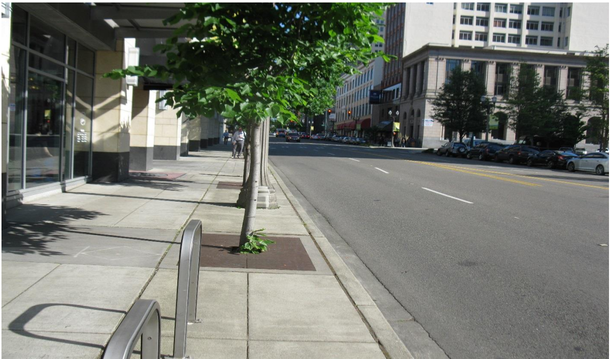
Photo 6: Soil Contamination Left-in-Place below the Sidewalk and Pacific Avenue – from the South
