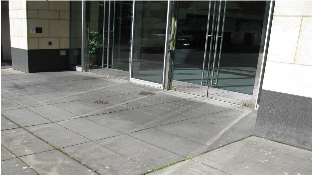
Photo 5: Pacific Plaza Garage Building, Soil Contamination Left-in-Place [in Front and under the Building (foundation columns) and below the Sidewalk] and Concrete Cap – from the Northeast
