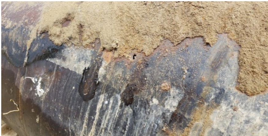
Photo 7: Hole in UST 1
