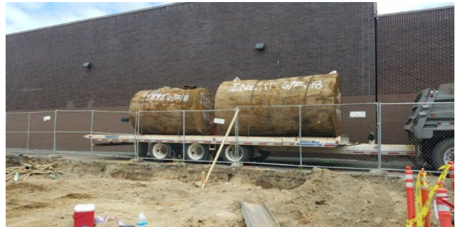
Photo 12: Secured and Labeled USTs
