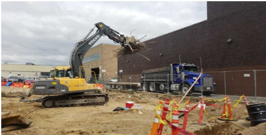
Photo 11: Loading Product Piping
