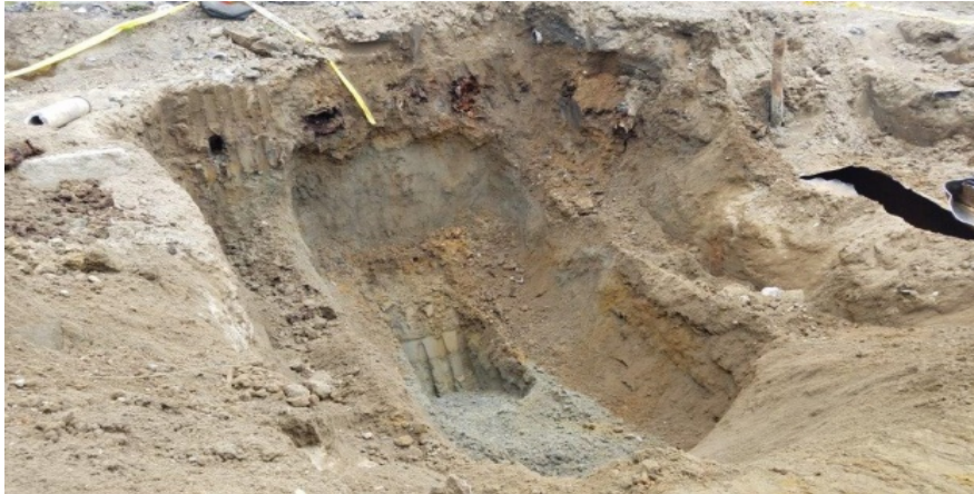
Photo 9: Stained Soil Beneath UST 4
