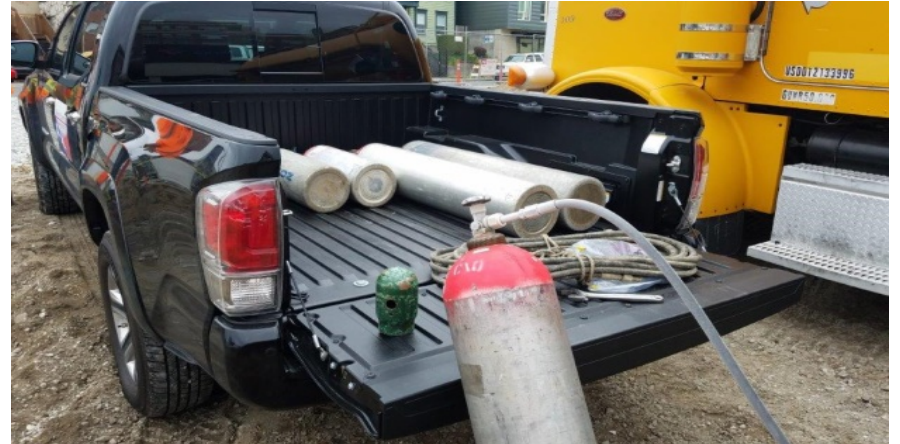
Photo 2: CO2 for Tank Inertion
