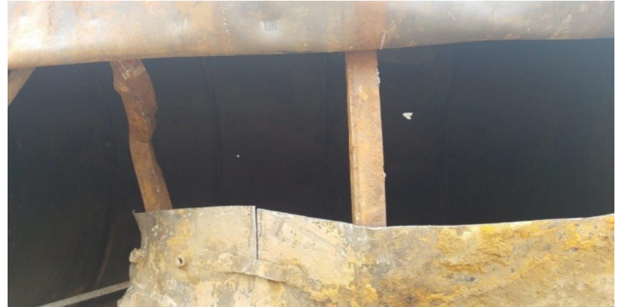
Photo 10: Holes in UST 4
