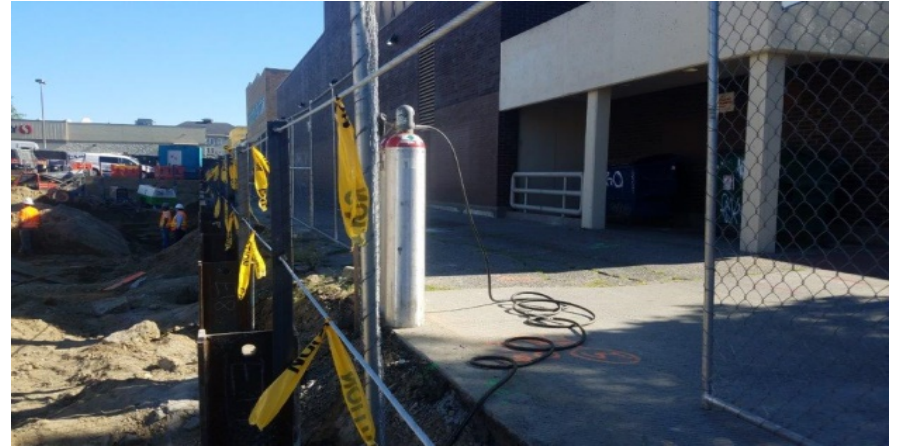
Photo 2: CO2 for Tank Inertion
