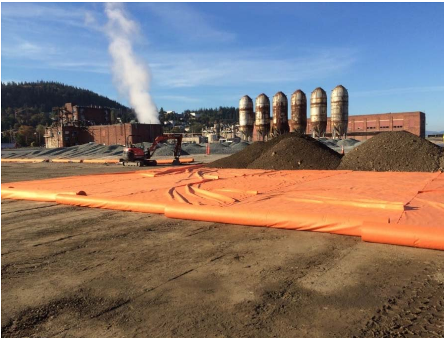
Photo 10. Separation geotextile placed over graded and compacted soil/veneer site-derived fill. Gravel borrow to be placed over geotextile.
