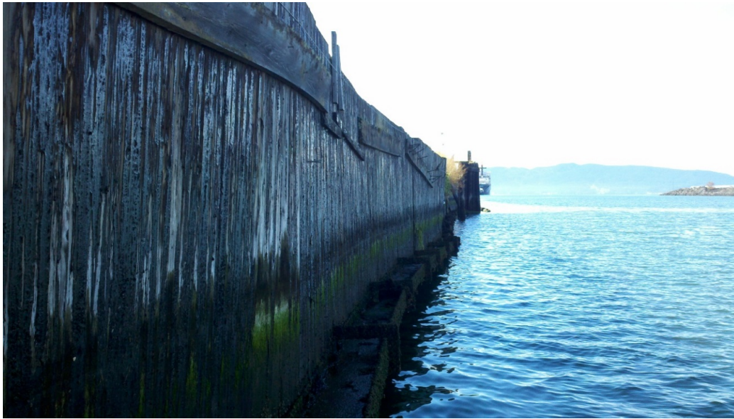
Before Construction: Most of the South Shoreline area consisted of a vertical creosote-treated timber bulkhead supporting an area of fill and the abandoned concrete clarifier structure.
