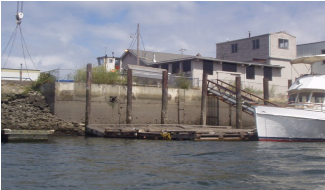
Before Construction: The shoreline was unstable with a damaged concrete bulkhead. Creosote-treated pilings and unauthorized floats were present in the offshore area.
