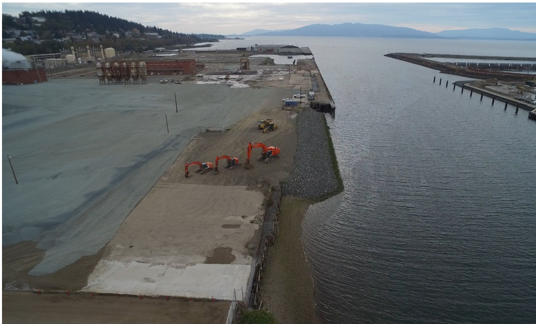
After Construction: Unused in-water structures were removed. The clarifier and associated creosote-treated timber bulkhead were removed. A shoreline cutback was performed to create a gently sloping, stable shoreline. The shoreline and subtidal areas were capped to safely contain residual impacted sediments.
