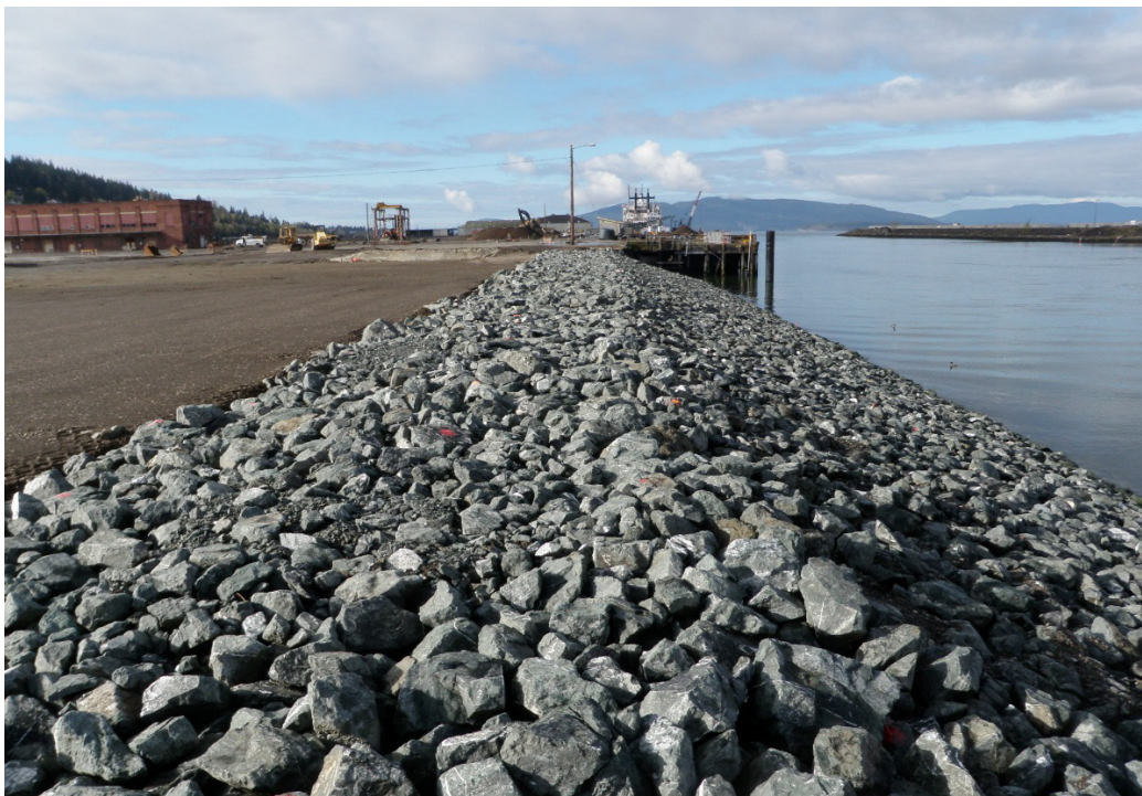
After Construction: The bulkhead in the South Shoreline area was removed along with the clarifier and other structures. The slope was cut back to provide a stable, sloping shoreline and enhance habitat quality and quantity in this area.
