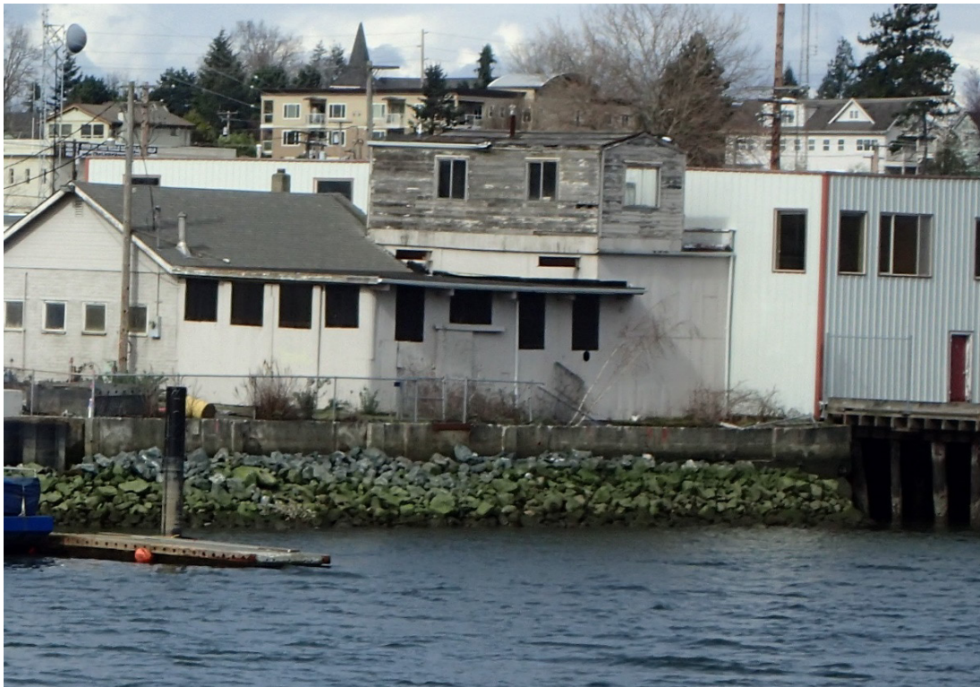
After Construction: The creosote-treated pilings and unauthorized floats were removed. The exposed bulkhead was eliminated and the shoreline was stabilized with a sloping engineered cap.
