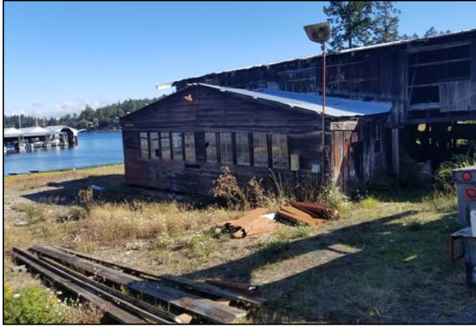
Photo 5. A view looking north at the old boat building structure. The building's condition made it unsafe to enter.
