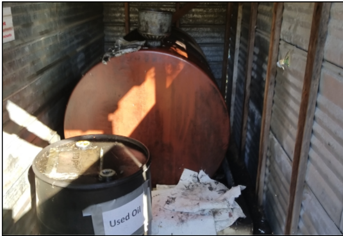
Photo 3. A view of a used/waste oil drum and AST in the southern portion of the oil storage building.
