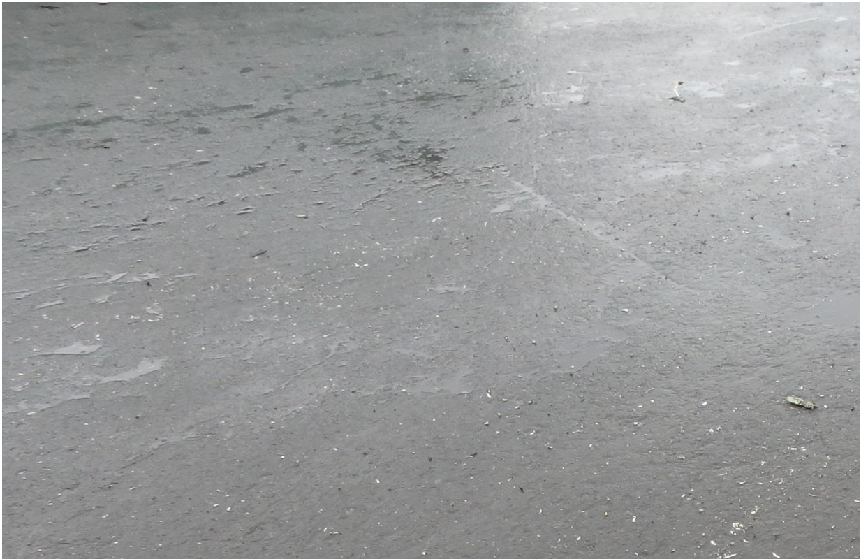
Figure 4. Gouges and debris on north area cap pavement surface
