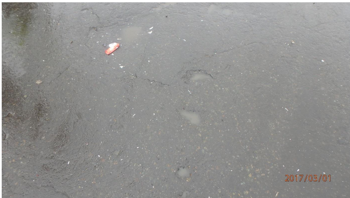
Figure 5. Gouges and debris on north area cap pavement surface
