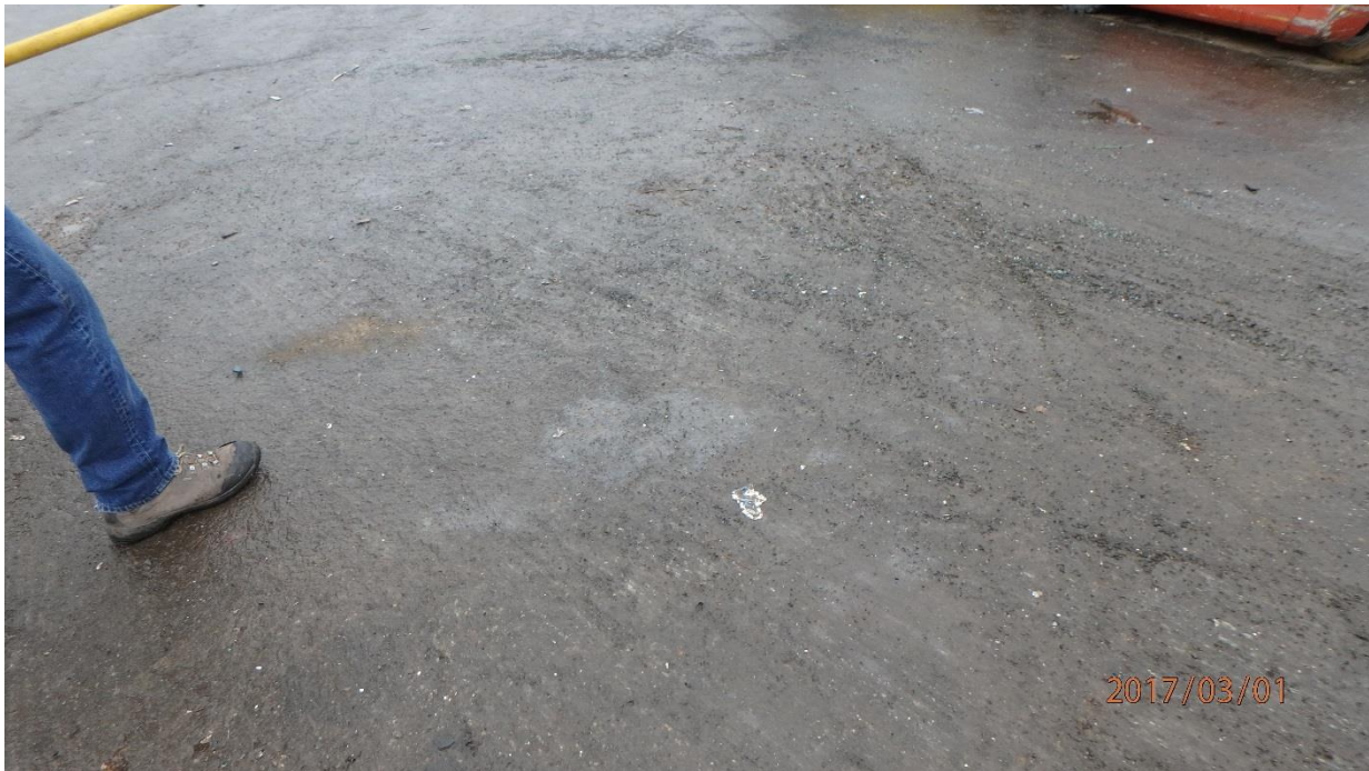
Figure 7. Loose gravel and debris resulting from surface raveling on north area cap pavement surface
