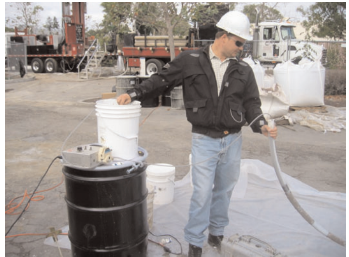
Figure 7 Pre-installation grouting of CMT by injection of grout through 1/4" (6 mm) tubing using a peristaltic pump.
