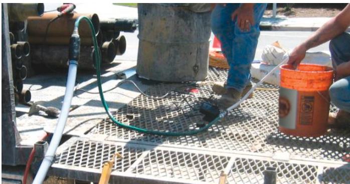
1" diameter Grout Line connected to Grout Adaptor, attached to bottom of CMT.
