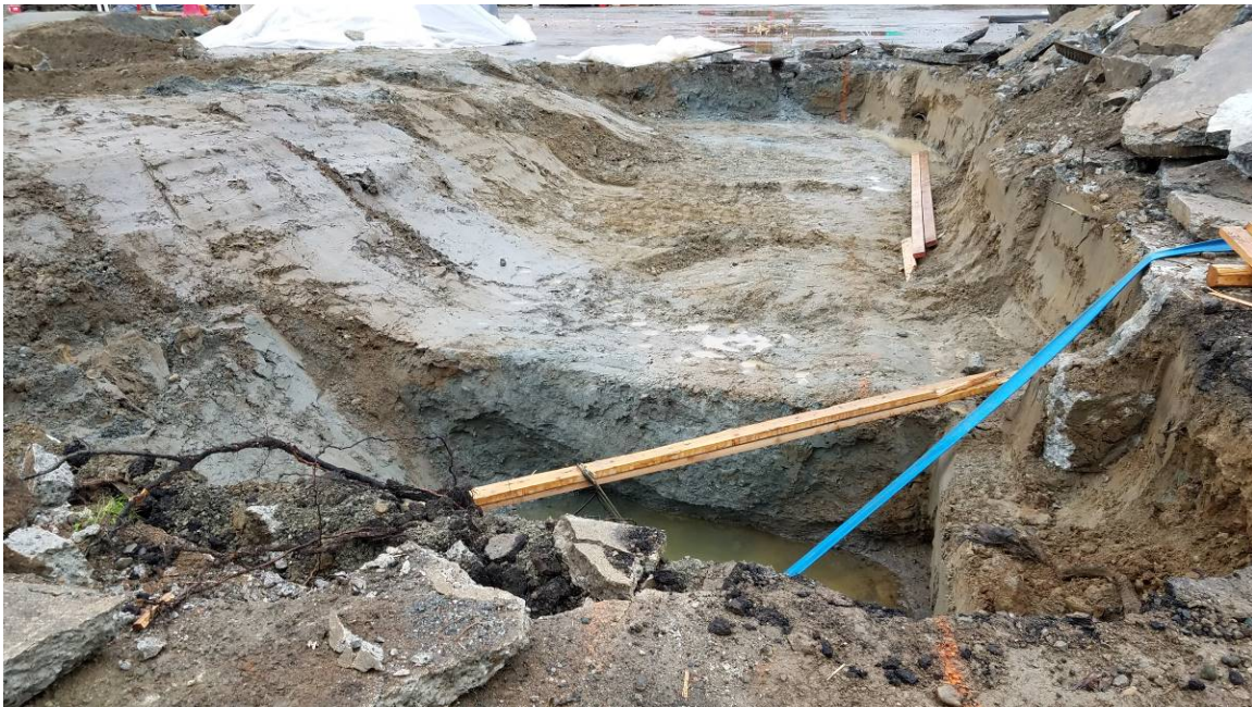
Photo 4. View looking north from the south end of the trench drain alignment in the former western service area. Sumps were initially installed at the ends of this excavation to collect water, which was pumped out for off-site disposal. June 2018.
