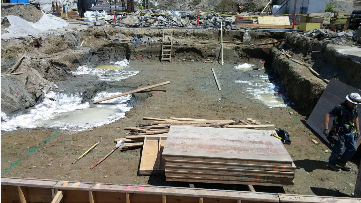
Photo 5. Looking east into the excavation for Mat Foundation Stair 1. ORC has been placed in over-excavated areas in the northeast and southeast corners and under where lifts were encountered in the north-central portion of the excavation. June 2018.
