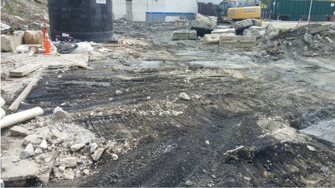
Photo 7. View looking south at the former eastern service area after removal of most of the concrete floor slab. Characterization sampling and field observations indicated that the gravel bedding layer was contaminated. July 2018.
