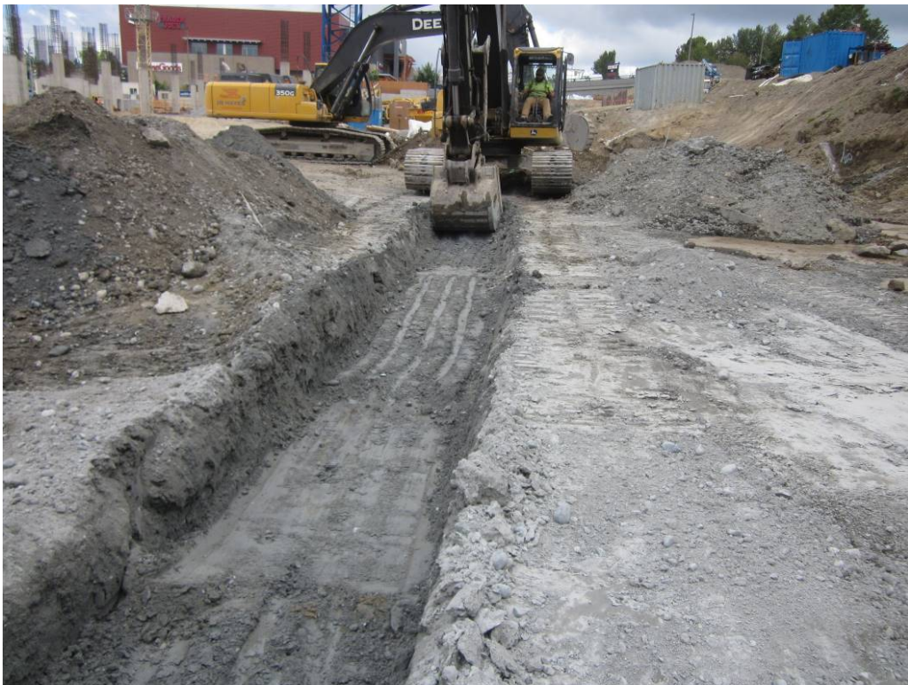
Photo 8. View looking north during over-excavation of the former trench drain alignment that had served the eastern service area. July 2018.
