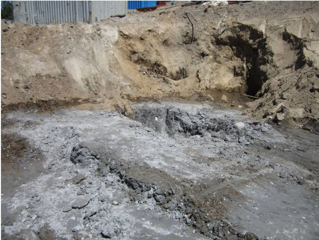
Photo 9. View of spot excavations in the northeast corner of the former eastern service area. Note that water is perched on the gray glacial till, which is dry. July 2018.
