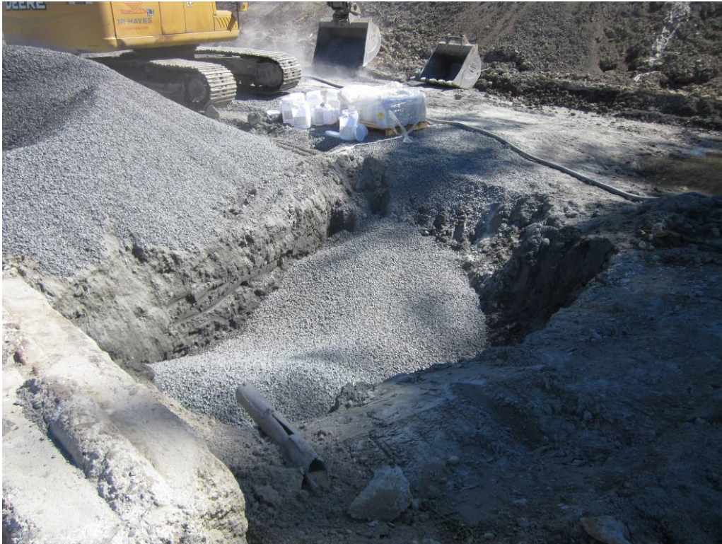
Photo 11. Backfilling an excavation in the southwest corner of the eastern service area (looking NE). The excavation was installed to remove an area of sandy fill. SCS suspects that the fill was placed after the removal of a waste oil UST in November 1988. July 2018.
