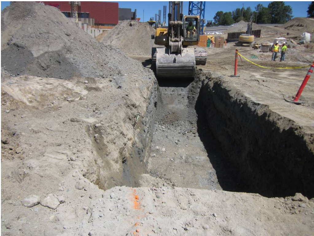
Photo 6. Looking north during over-excavation of the northern portion of the former trench drain alignment that had served the western service area. July 2018.
