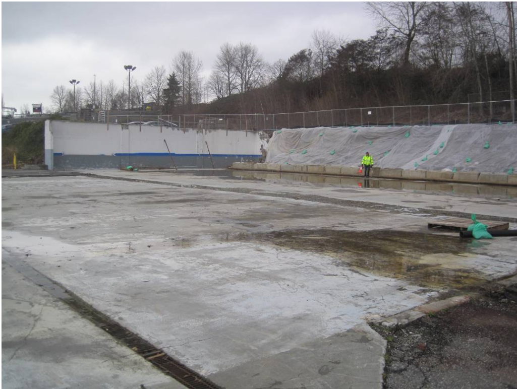
Photo 2. View looking northeast from the south side of the western service area. Note the trench drain in the left foreground.
