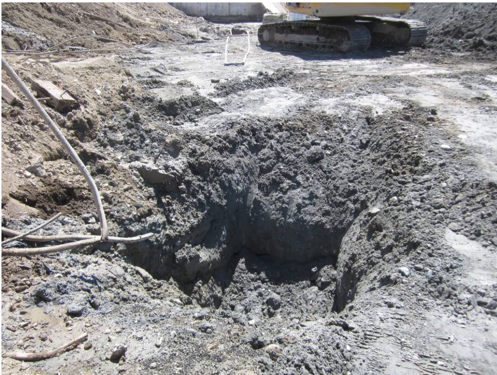
Photo 10. View of the excavation installed to remove a dual-cylinder hydraulic lift from near the northeast corner of the eastern service area (R16). No groundwater was identified within the gray till. July 2018.
