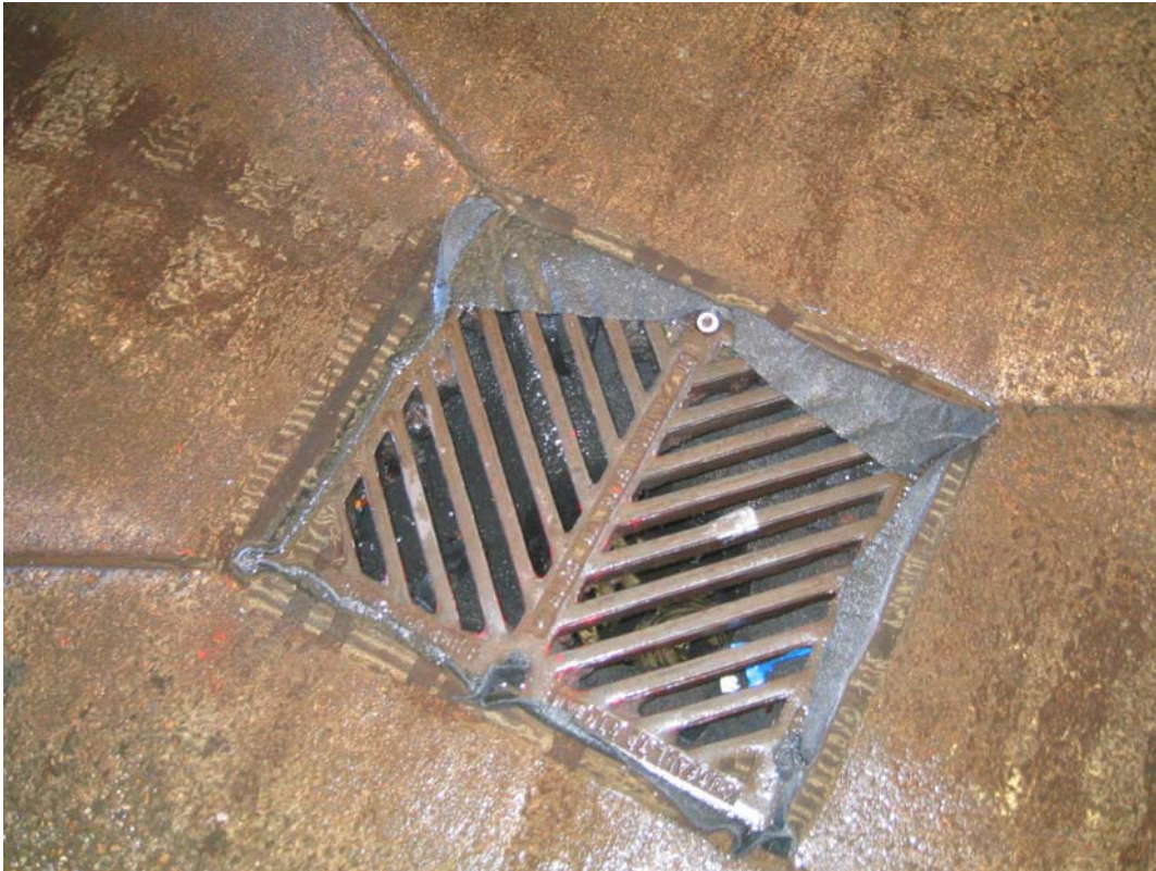
Photo 5. View of a sediment filter installed in the storm-catch basin at the wash rack at Eastside Chrysler-Jeep. Each of the storm drains at 126 116 th Avenue NE has a sediment filter installed.
