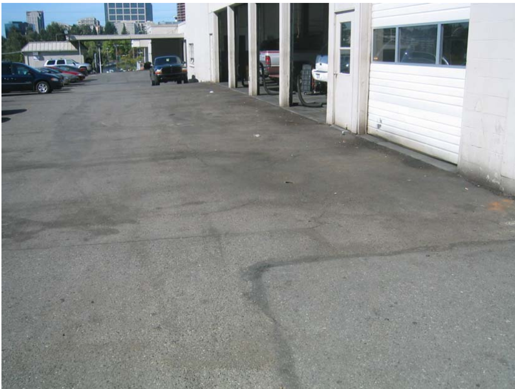
Photo 14. View looking west along the south side of the Dodge of Bellevue service bays. Note the staining on the pavement. Staining low on the walls and doors is also apparent, likely from water splashing oily dirt onto the vertical surfaces.
