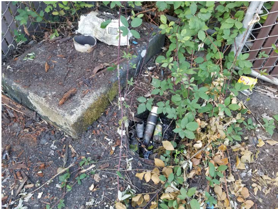
Photograph 6: Hole with piping with standing oil.
