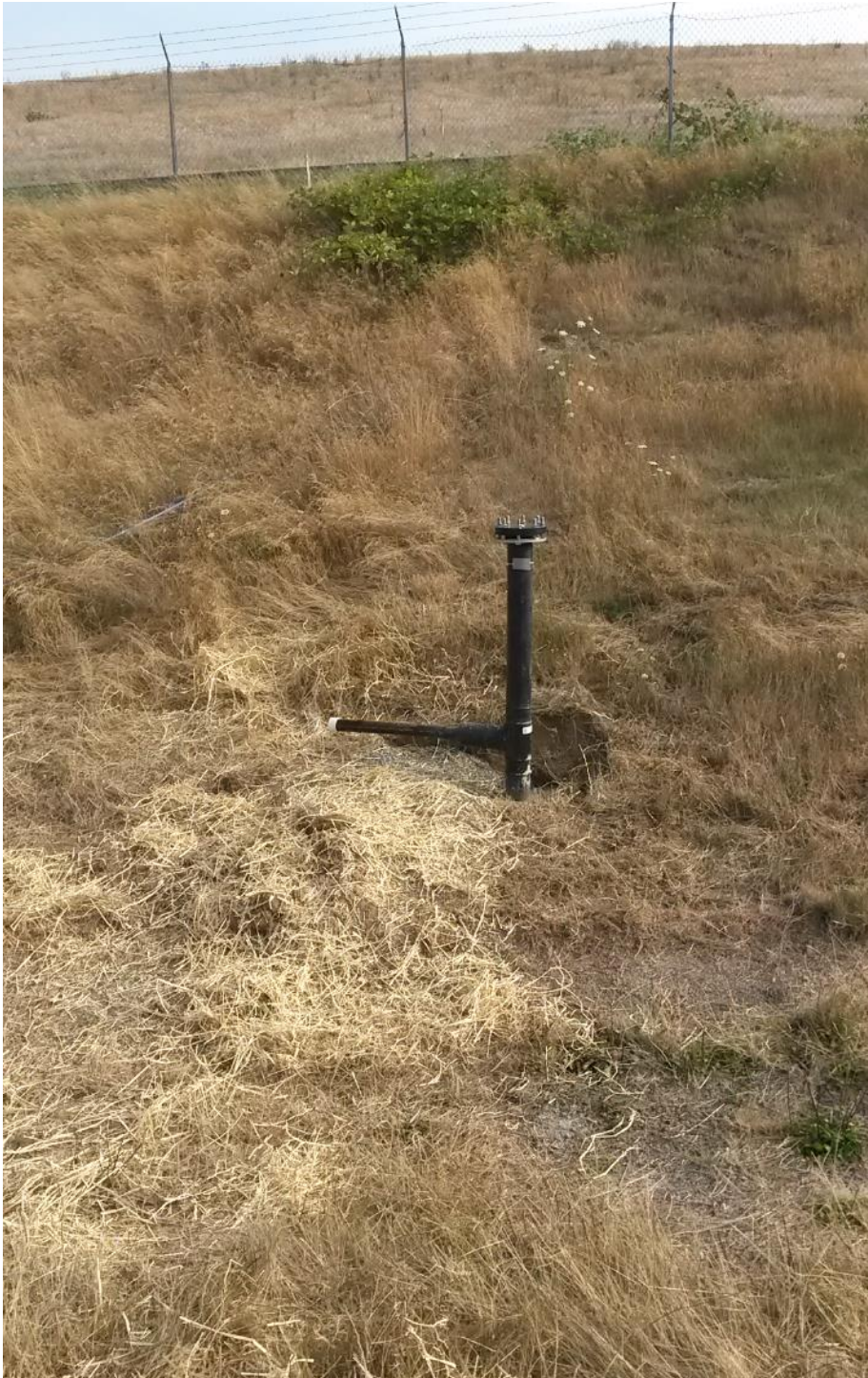
Photograph 1. Gas extraction well GW-9, completed before connection to gas collection system
