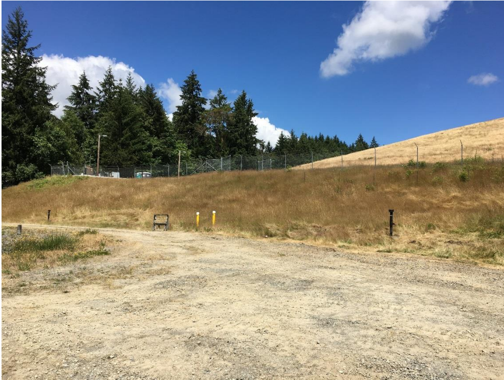
Photograph 1. View facing northwest showing newly installed LFG extraction wells (black stick-ups) GW-10 (right) and GW-11 (left).
