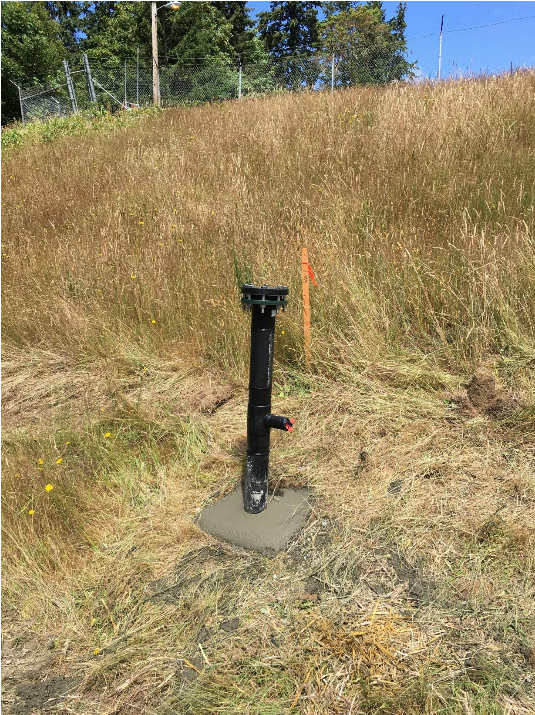
Photograph 3. View of completed extraction well GW-11 facing northwest up-slope. The 2-inch tee fitting is facing east along the topographic contour of the hill.
