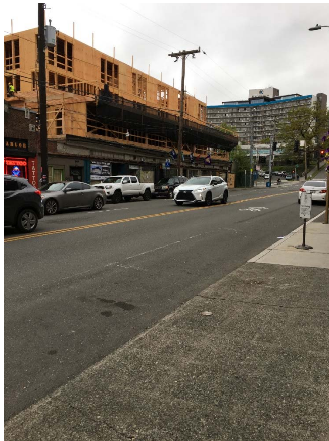
Eastern side of the Bungalows with construction visible above first floor retail. The main building of the Bayview residential community is visible in the background. (taken from across Queen Anne Ave N)
