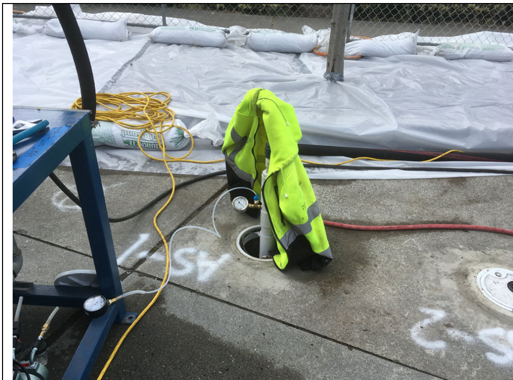
Photo #12: Well attachment at AS-1 with two pressure gauges attached.
