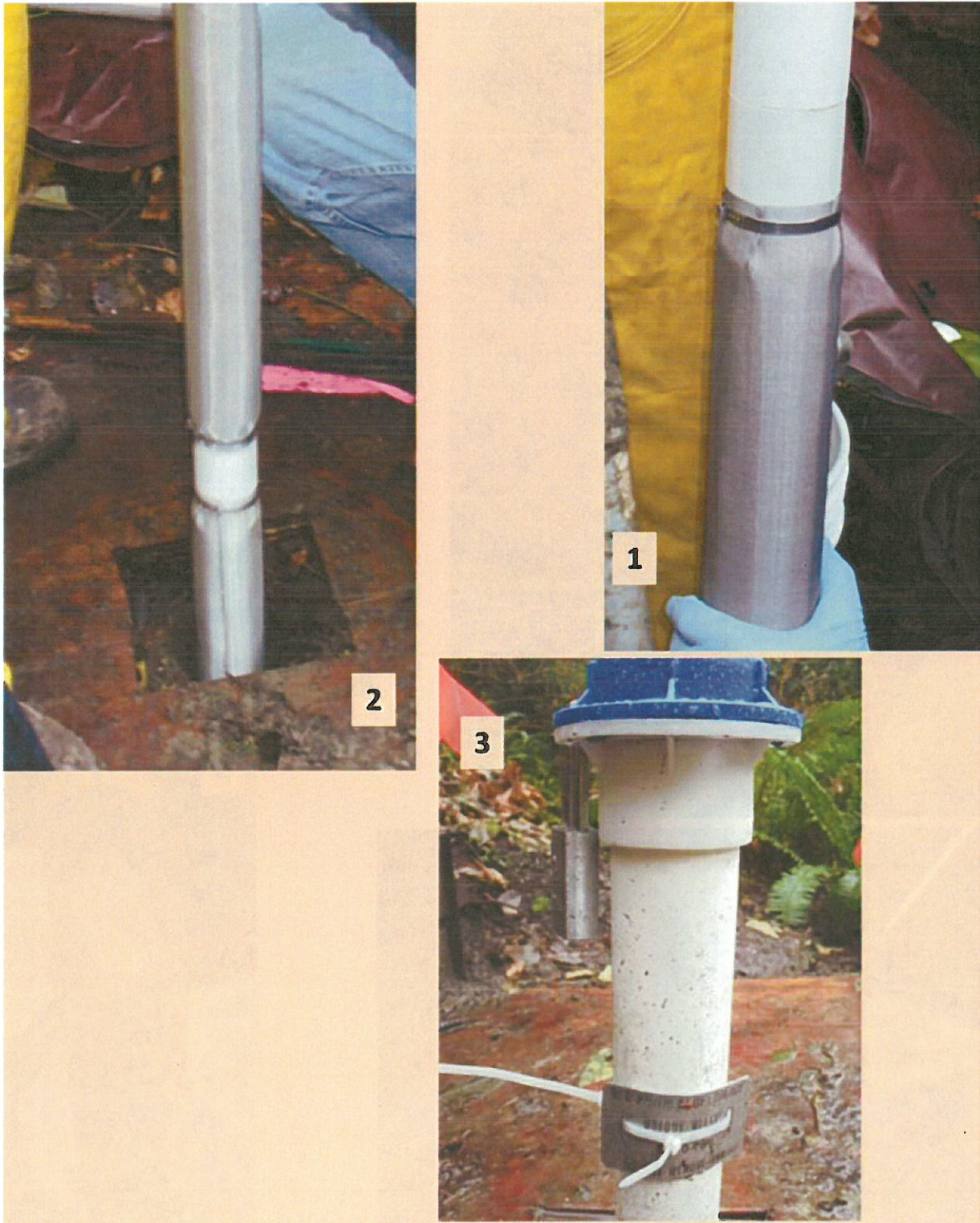
(1) Pre-packed screen around 0.010-inch slots on 2-inch PVC tubing (2) Placing two five-foot pre-packed screens (and 0.010-slots) into borehole (3) Well locking cap, lock and state well tag.
