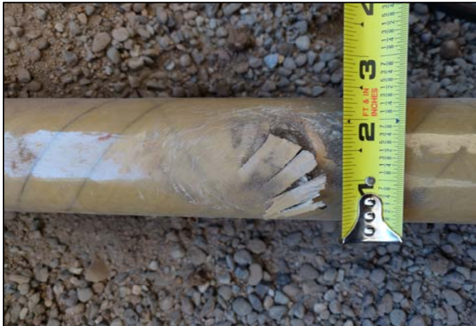
Photo 3. A closeup view of the ruptured product line showing the delaminated fiberglass caused by contact with the hand auger.
