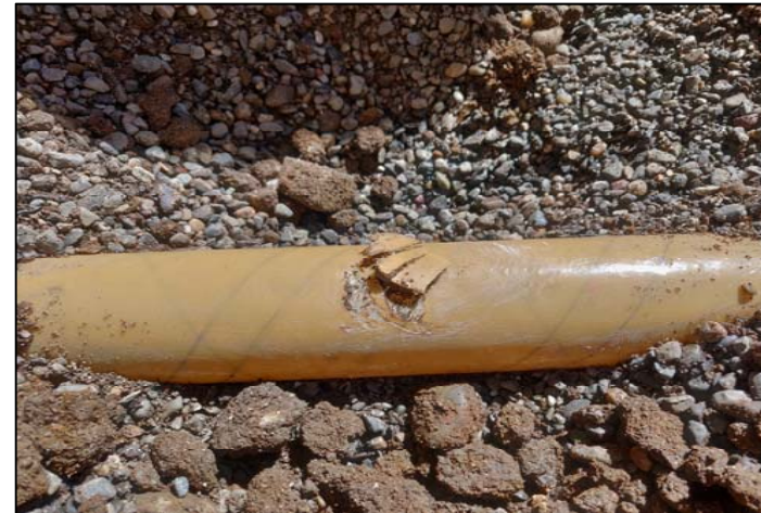
Photo 4. A closeup view of the ruptured product line. Note the auger scrape marks atop the product line.
