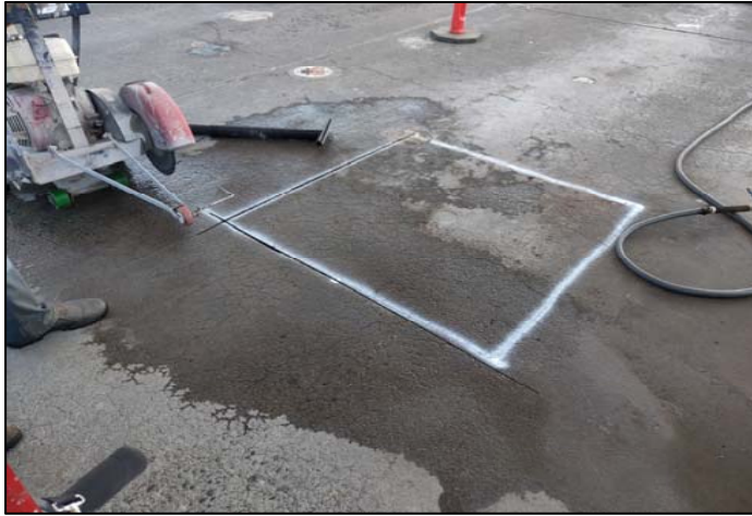
Photo 1. A view towards the northeast looking at the concrete cut with the northern HydroCon boring at the center.
