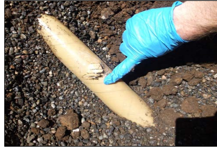
Photo 2. A view of the ruptured product line when it was first uncovered. Note the visibly stained pea gravel around the pipe.
