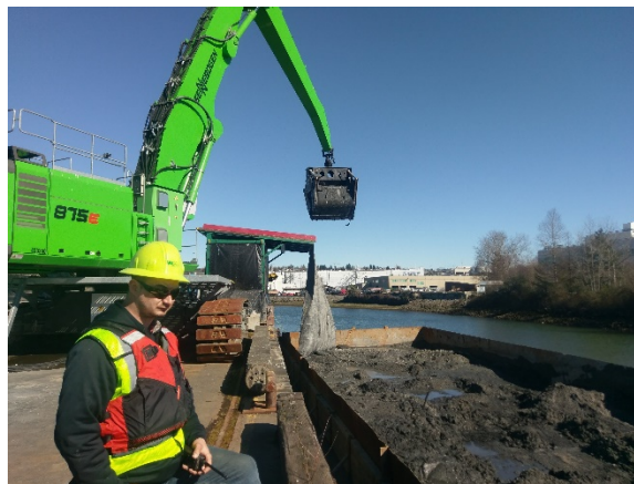
Exhibit 12. Sediment transloader at Duwamish Transfer Facility
