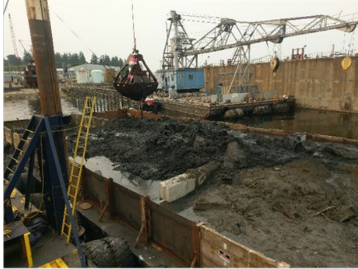
Exhibit 8. A digging bucket used during the Interim Action for portions of the dredge cut with larger woody debris present.
