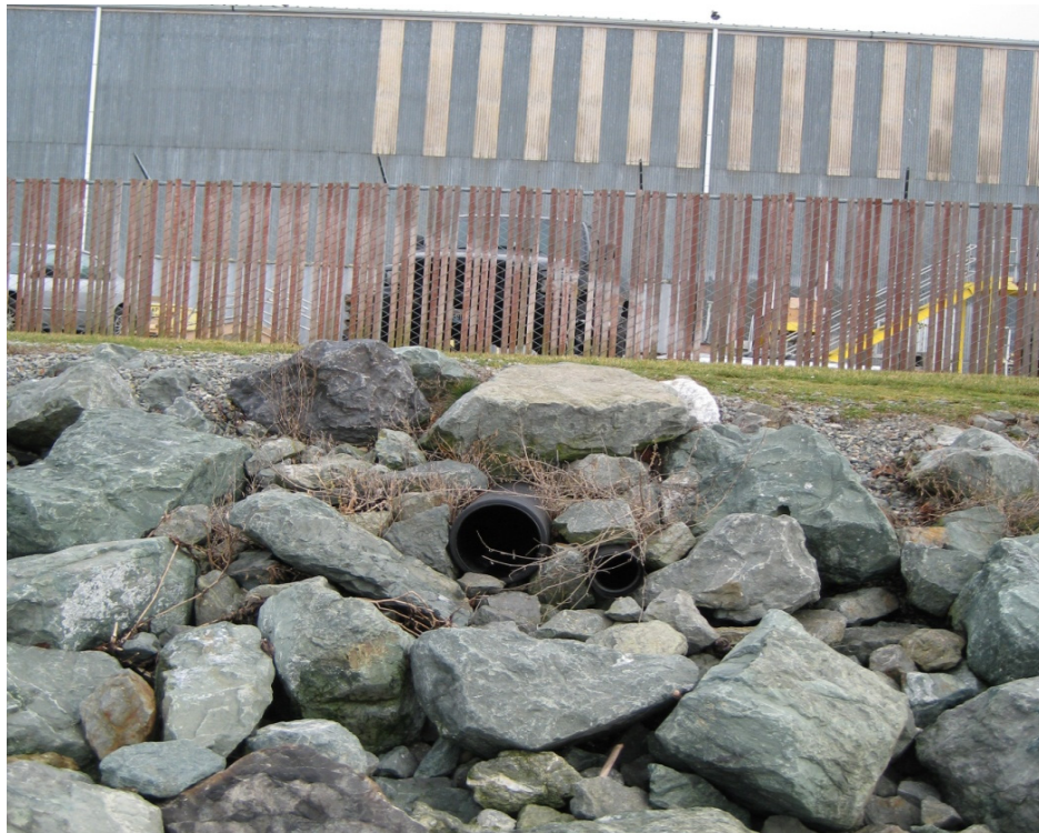
Photograph 14. Stormwater outfall pipe (left) and unused pipe (right) on riprap slope located along the western shoreline, January 2013.
