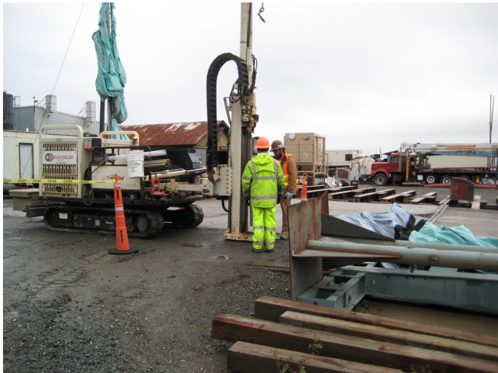
Photograph 8. Limited access Geoprobe setup for sampling to east of the Marine Railway Area at Location FS-21, January 2013.
