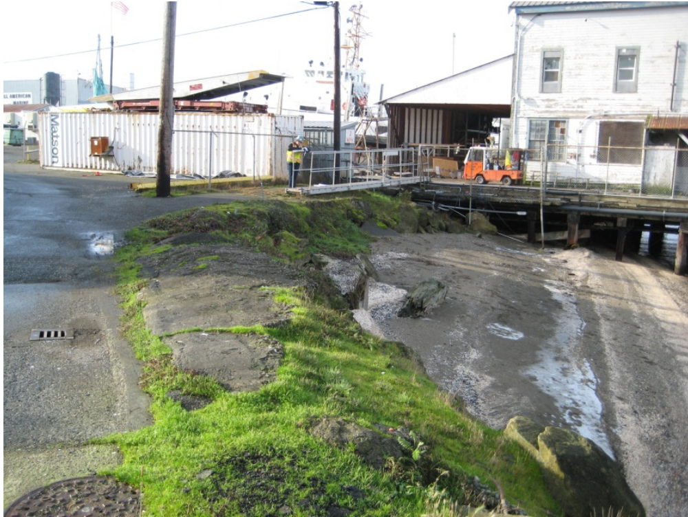
Photograph 7. View of pocket beach and stormwater catch basin located east of the main pier, January 2013.
