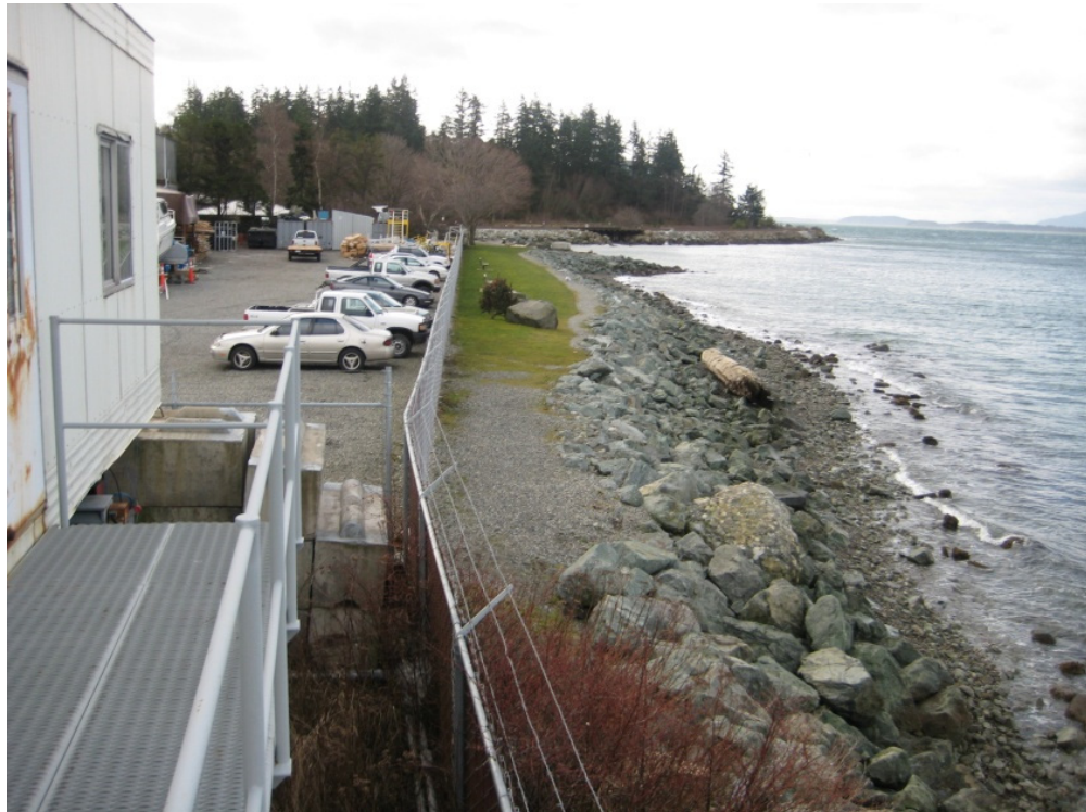
Photograph 6. View of the western shoreline riprap slope and adjacent park area, March 2011.
