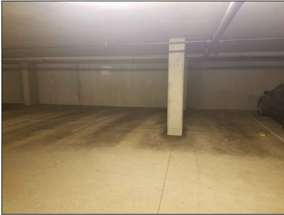
Photograph 1: View looking west representing the condition of the garage floor slab in Area 1.
