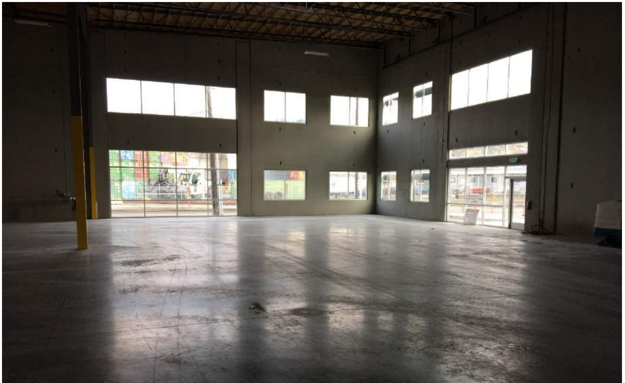
Photograph 12. NE Office Node of Building A. Passive Vapor Mitigation system located under slab.
