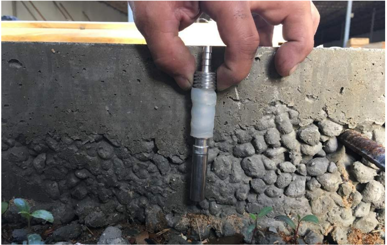
Photograph 13. Typical Vapor Pin installed in Building A and B.
