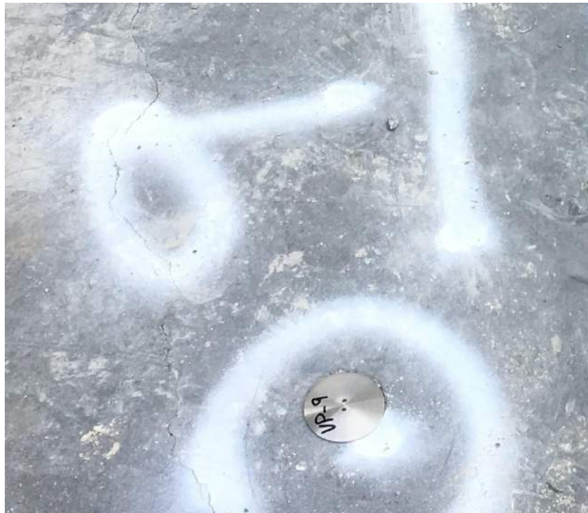
Photograph 4. Vapor pin with flushed-cover.
