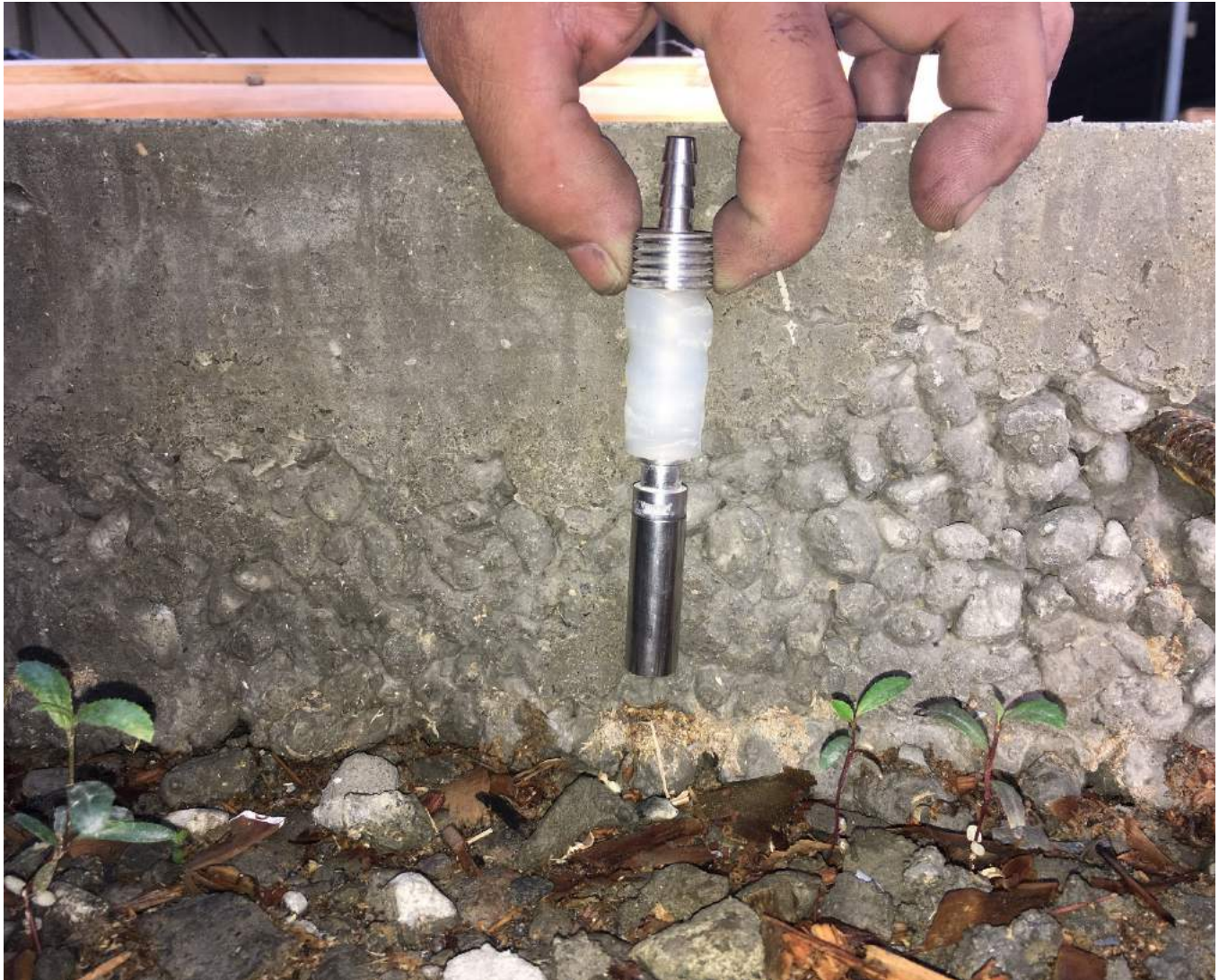
Side view of the slab in Building A with Vapor Pin for scale.
