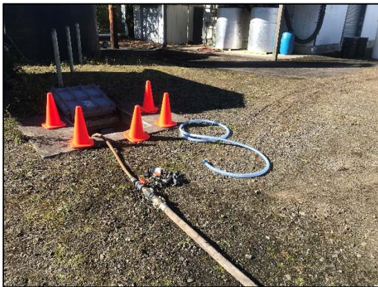
Photo 3: Direct water source – fitted for fire hose to RRS trailer tanks.
