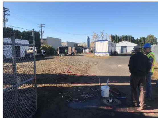
Photo 6: Monitoring well water flush – added compression fitting and pressure gauge.
