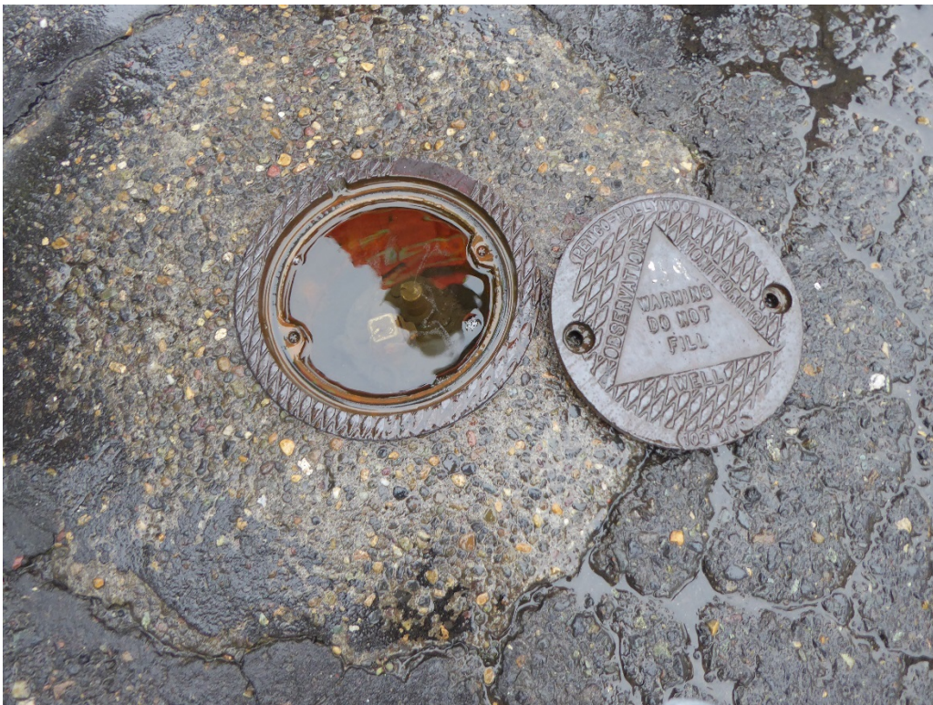
Monitoring well on Linde property
