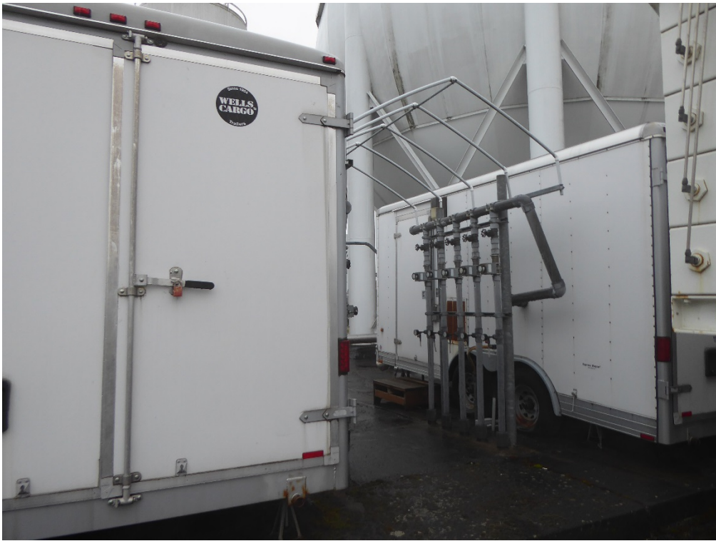
Soil vapor extraction and in-well stripping systems (now shut down) on Linde property
