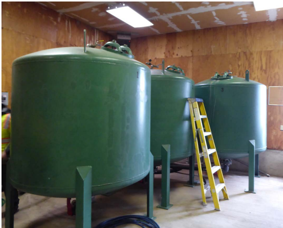
Ion exchange tanks
