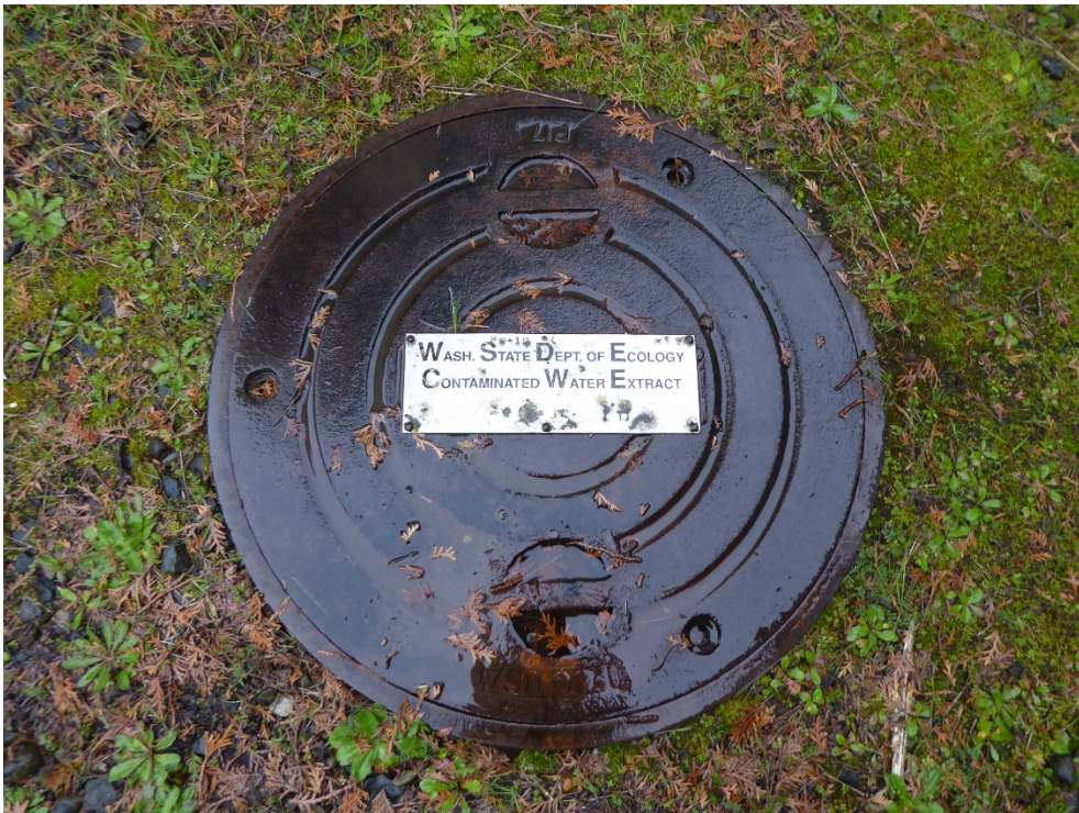
Extraction well PW-1
