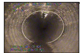
DEFORMED PIPE AT 20 FT FROM CB26
