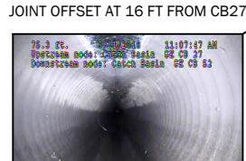
SAGGED PIPE AT 75 FT FROM CB27
