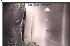
CRACK ON PIPE AT 55 FT FROM CB12
