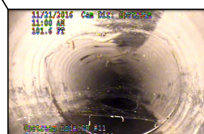
DEFORMED PIPE AT 102 FT FROM CB12
