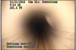
DEFORMED PIPE AT 204 FT FROM CB6
