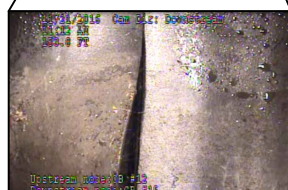
CRACK ON PIPE AT 55 FT FROM CB12
