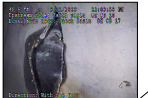
FRACTURE AT 41 FT FROM CB18
