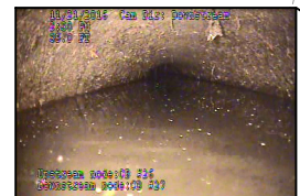
SAGGED PIPE AT 35 FT FROM CB26
