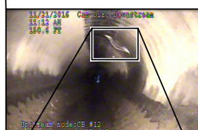
CRACK ON PIPE AT 154 FT FROM CB12
