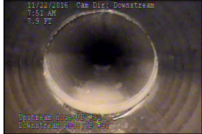
PIPE JOINT OFFSET AT 11 FT FROM CB31
