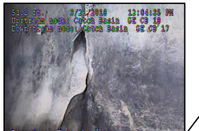
FRACTURE AT 51 FT FROM CB18
