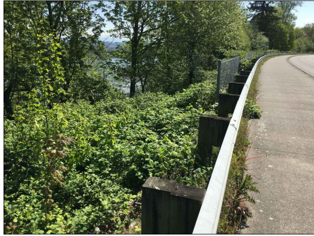
P-1 CF-2 VIEW SOUTHEAST: NORTH END OF EXISTING 4-FT CHAIN LINK FENCE
