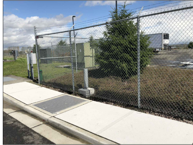
P-2 CD-2 VIEW NORTHEAST - NORTH POND PUMP STATION AREA
