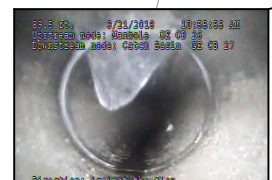
BROKEN PIPE AT 90 FT FROM CB27
