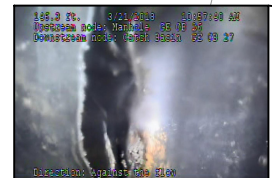
FRACTURE ON PIPE AT 146 FT FROM CB27
