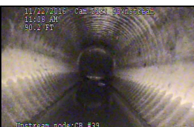
SAGGED PIPE AT 90 FT FROM CB39
