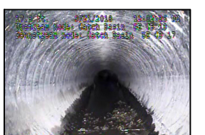
SAGGED PIPE AT 18 FT FROM CB18
