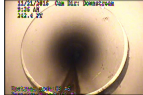
JOINT OFFSET AT 242 FT FROM CB6
