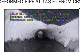
DEFORMED PIPE AT 199 FT FROM CB27
