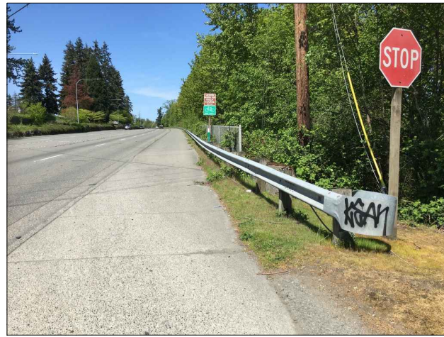
P-6 CF-2 VIEW NORTHWEST - SOUTH END OF GUARDRAIL AND 4-FT CHAIN LINK FENCE
