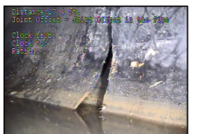
JOINT OFFSET AT 27 FT FROM CB18
