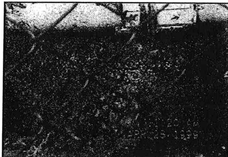
Below Clean Out - Leaking Piping System
