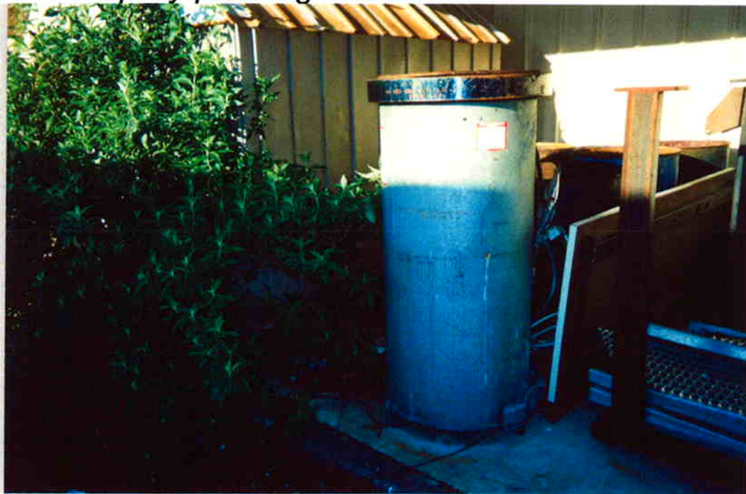
Photo 10: Empty solvent tank located along the east end of the main building.
