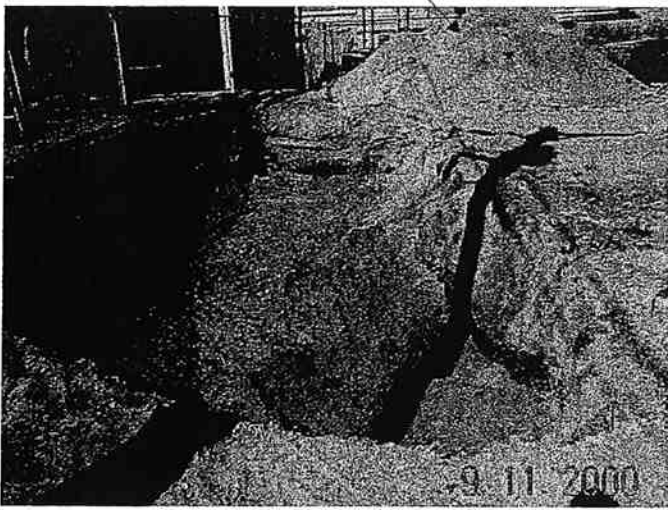
View the 0-4' BGS stockpile and excavation from the south, with excavation in the foreground..
