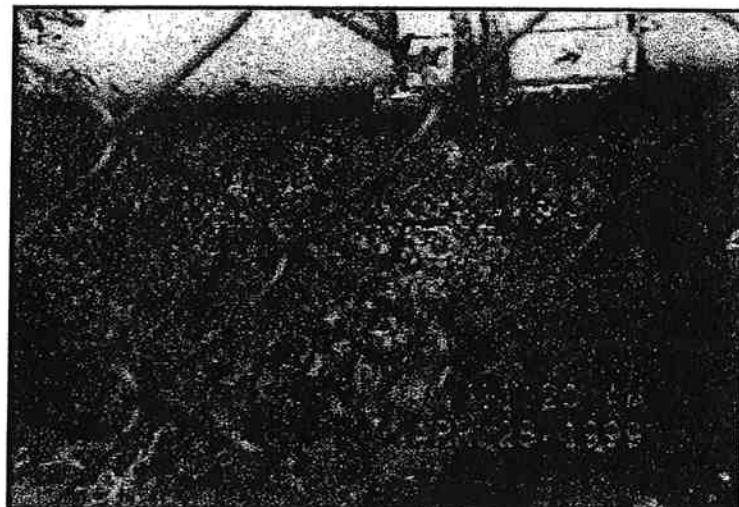
Below Clean Out - Leaking Piping System
