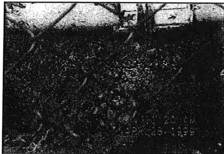
Below Clean Out - Leaking Piping System
