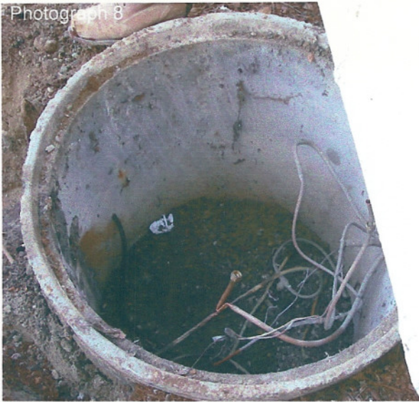
Piping system located inside concrete housing
