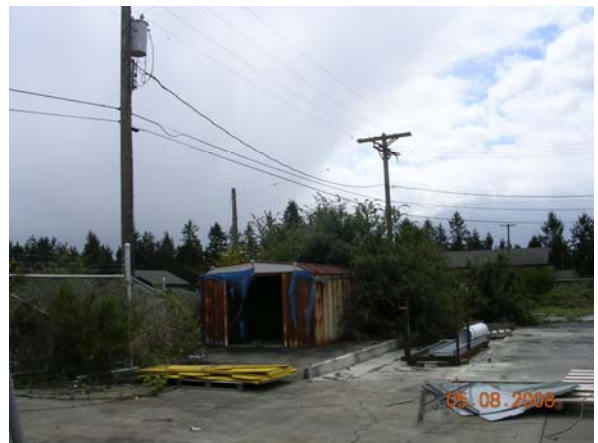
Photo #6 The paint storage building and a power pole with a transformer
