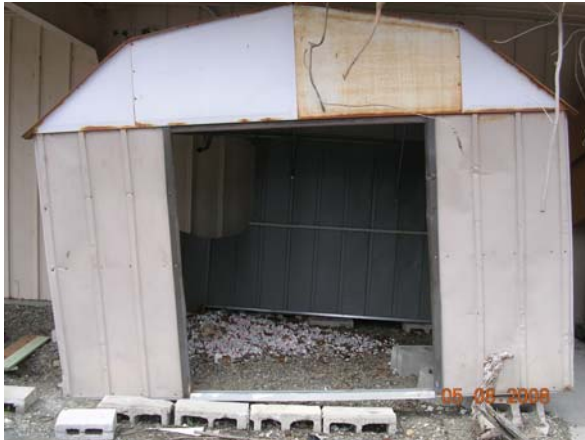
Photo #7 The battery storage shed
