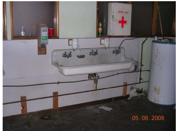
Photo #14 One of the sinks connected to the septic system
