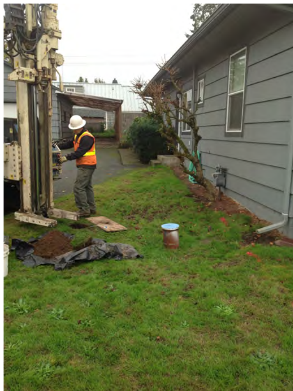
Photograph 12. Installing a soil gas sampling port outside the residence at 304 N 1st Avenue, November 2012.
