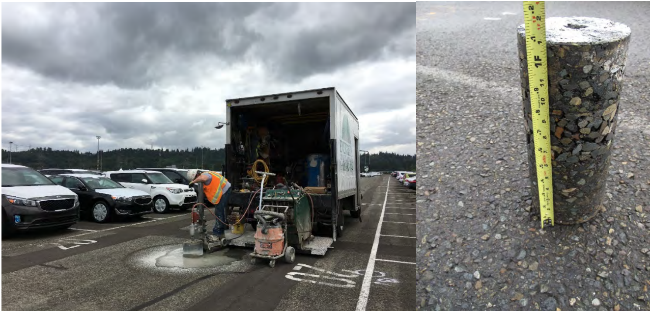
Photo E-1: Illustrates the double layered roller compacted concrete (RCC) and asphalt overlay that constitutes the Log Yard cap.
