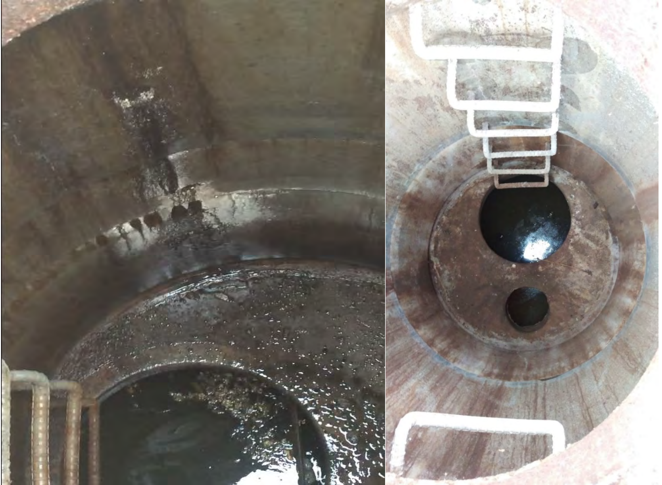
Photo E-11: Leakage observed in spill containment vault in February 2017 (Event 4; left). No leakage observed in spill containment vault in August 2016 – (Event 2; right)
