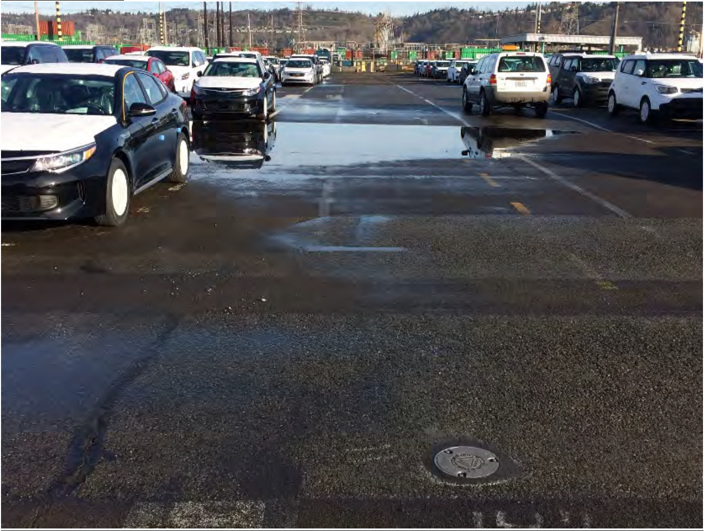
Photo E-8: TB-9: Ponding observed on the Log Yard Cap, looking north from monitoring well MW-11 (seen in foreground)
