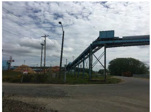
Pole-mounted transformers – facing east
