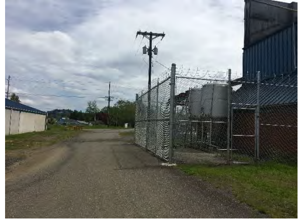
Pole-mounted transformers - facing east
