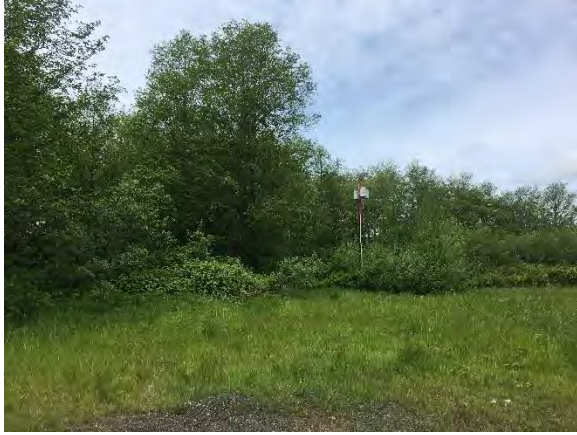
Pole-mounted transformers - facing west
