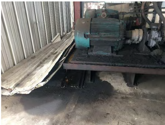
Equipment with oil staining inside Willis Enterprises warehouse
