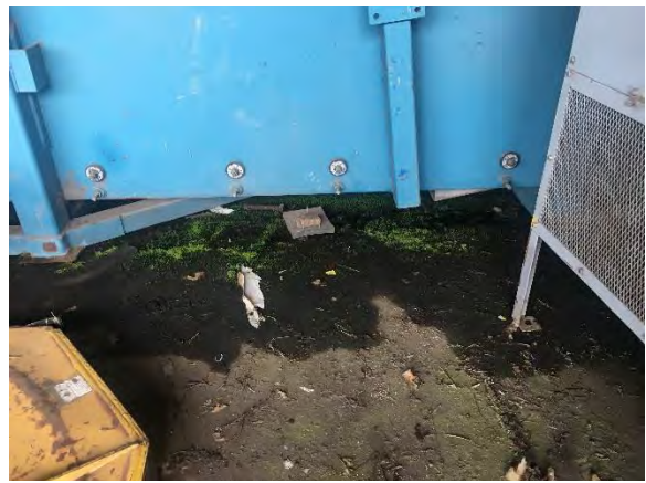
Oil staining inside Willis Enterprises warehouse – facing south
