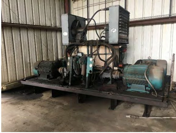
Equipment inside Willis Enterprises warehouse
