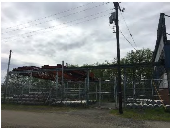
Pole-mounted transformers - facing south
