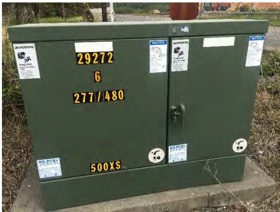
Pad-mounted transformers – facing north
