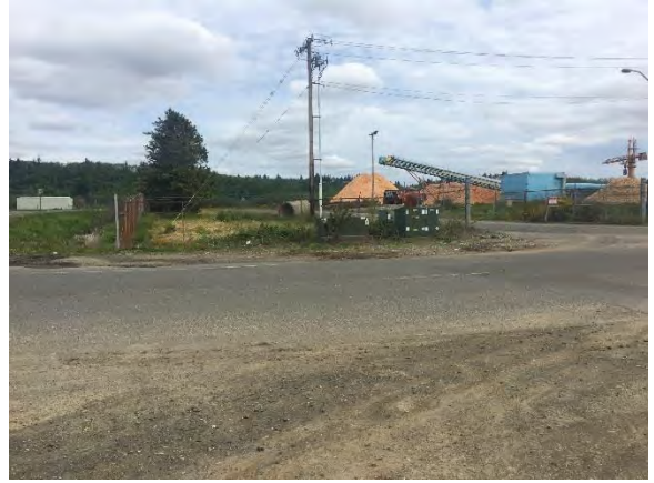
Pad-mounted transformers – facing north
