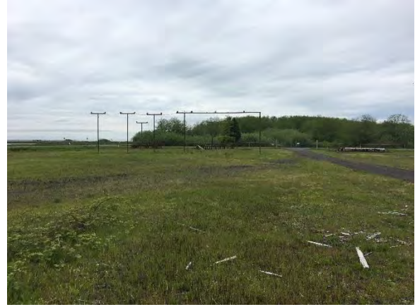
View of airport lights located on west/northwest portion of property - facing west
