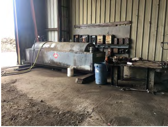
Diesel AST with oil staining
