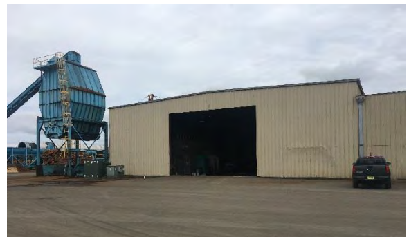
Pad-mounted transformers – facing north
