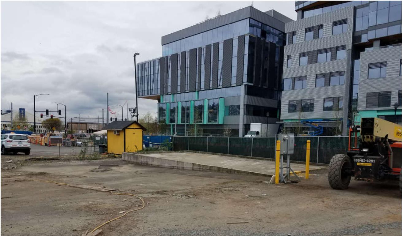
Photograph 11: View to the northeast – Former system compound area following completion of system removal.
