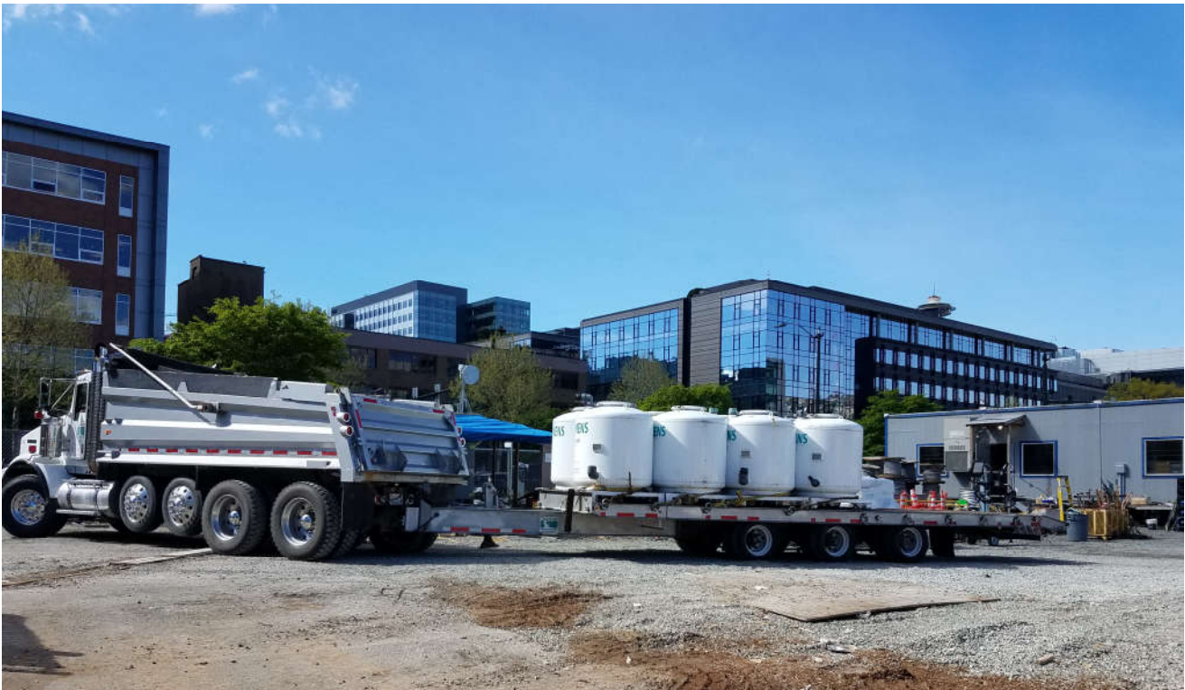
Photograph 8: View to the southwest – Carbon vessels loaded onto trailer for removal from site.
