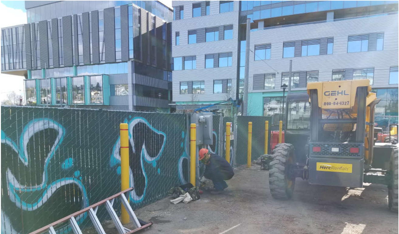
Photograph 3: View to the east – Electrician performing power disconnect at main system breaker.
