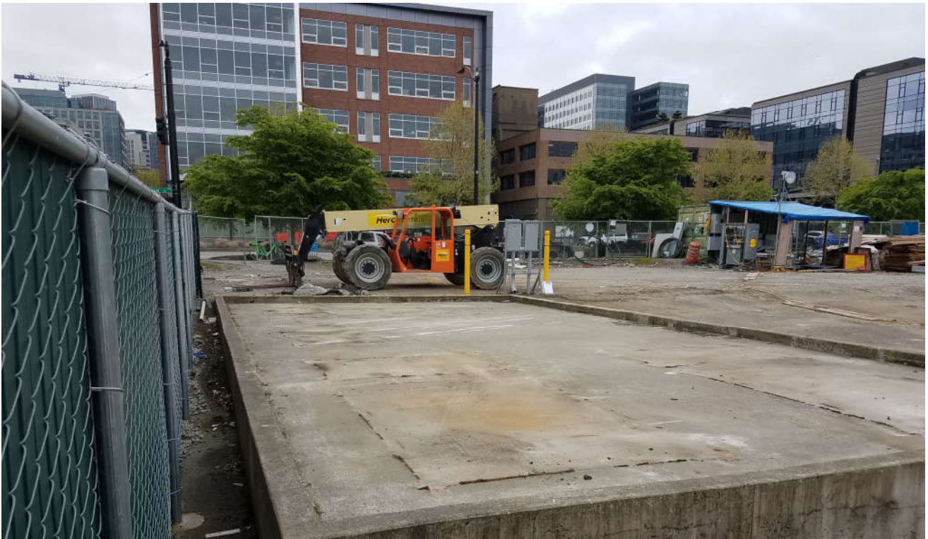
Photograph 12: View to the south – Former system compound area following completion of system removal.
