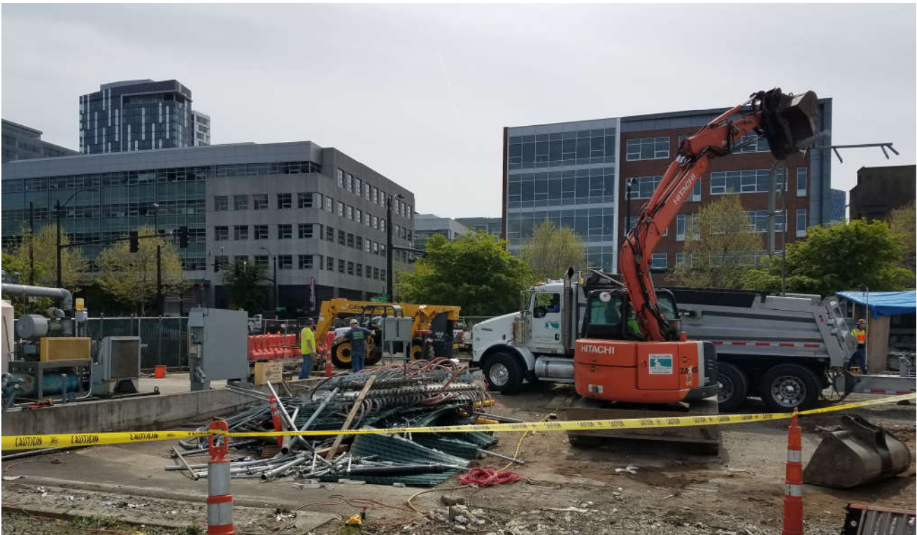
Photograph 10: View to the south – Loading system materials to truck for off site disposal.
