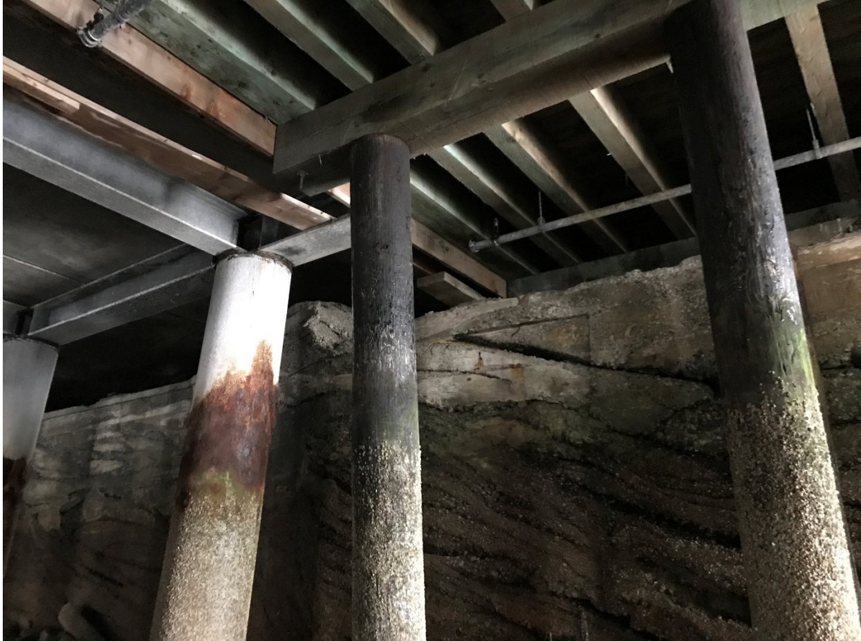
Under-wharf view close up of bulkhead and wharf interface near the west end of the wharf.
