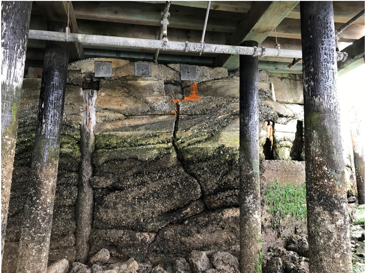
Under-wharf view of the southwest bulkhead on Curtis Wharf. Pipe is for fire suppression system. No evidence of historical product lines coming through the bulkhead.
