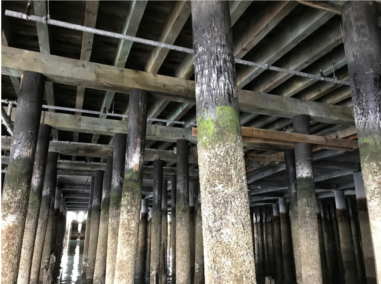
Under-wharf view from the bulkhead looking north. Pipe is for fire suppression system.
