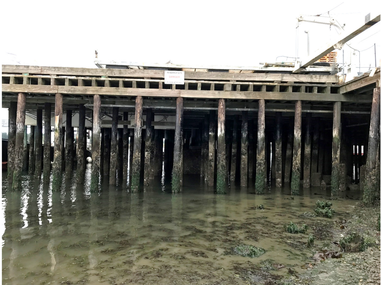
View of the southwest section of Curtis Wharf from the lower beach.
