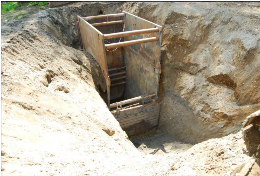
Photograph 4: May 12, 2011 - Looking southwest as the excavation of the north cell is reaching approximately 25 feet bgs.
