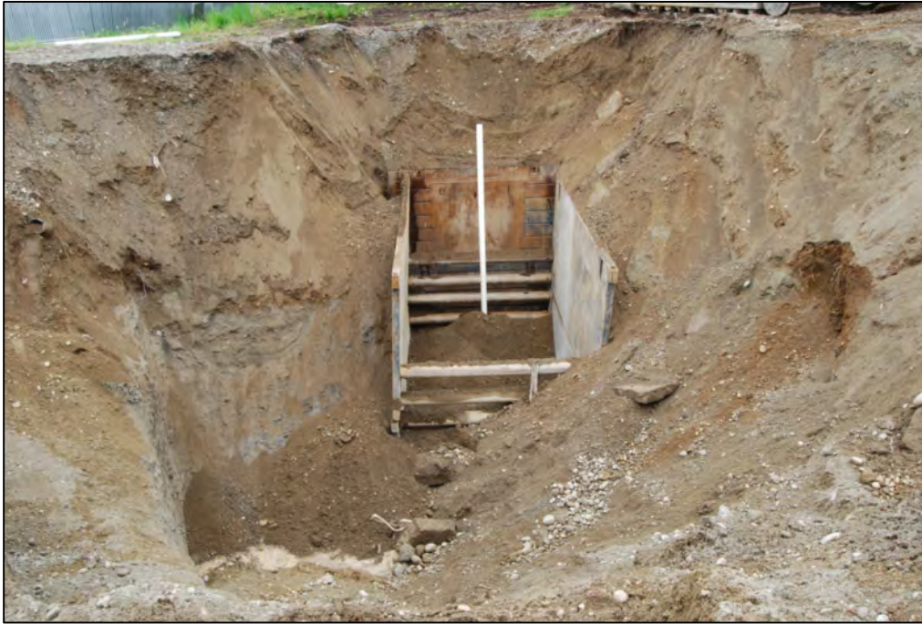
Photograph 9: May 16, 2011 - Looking south, photograph showing the final shape of the remedial excavation.
