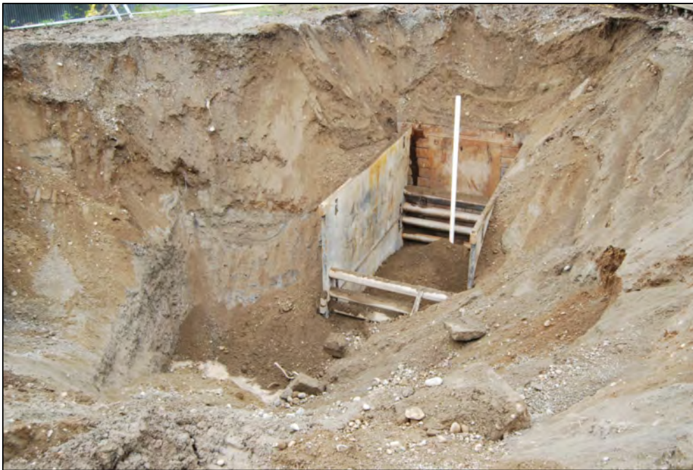
Photograph 8: May 16, 2011 - Looking southeast, photograph showing the final shape of the remedial excavation.
