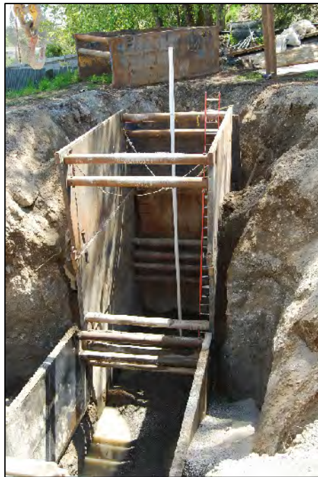
Photograph 6: May 13, 2011 - Looking south across the remedial excavation with shoring and stand pipe in place.
