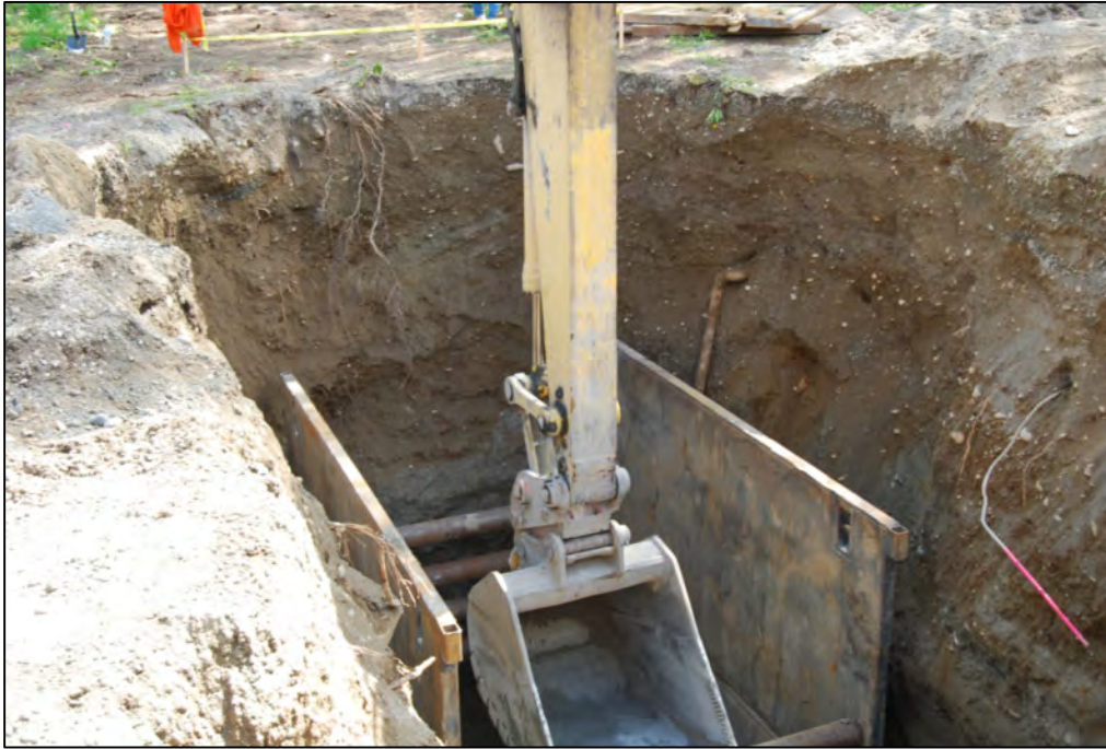
Photograph 1: May 10, 2011 - Looking southwest at the southern half of the excavation. Note the pipe in the sidewall that was related to the UST system.
