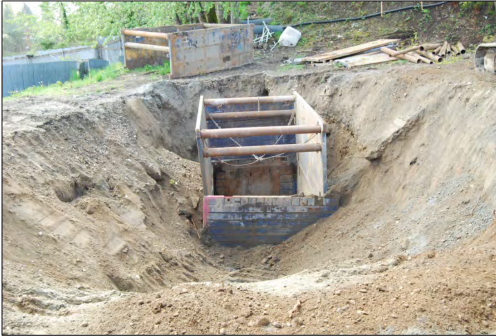
Photograph 3: May 12, 2011 - Looking south across the remedial excavation. The north cell excavation has been started.
