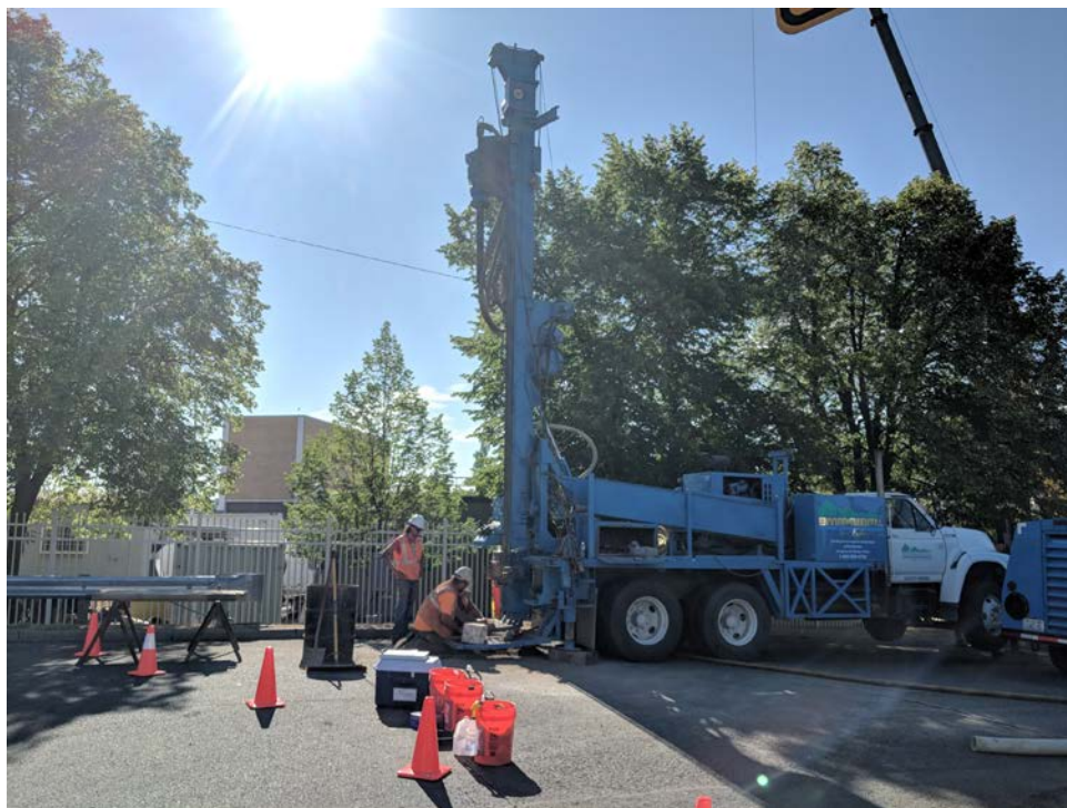
Environmental West Exploration drilling monitoring well MW-1A using air rotary drilling. (view looking east)
