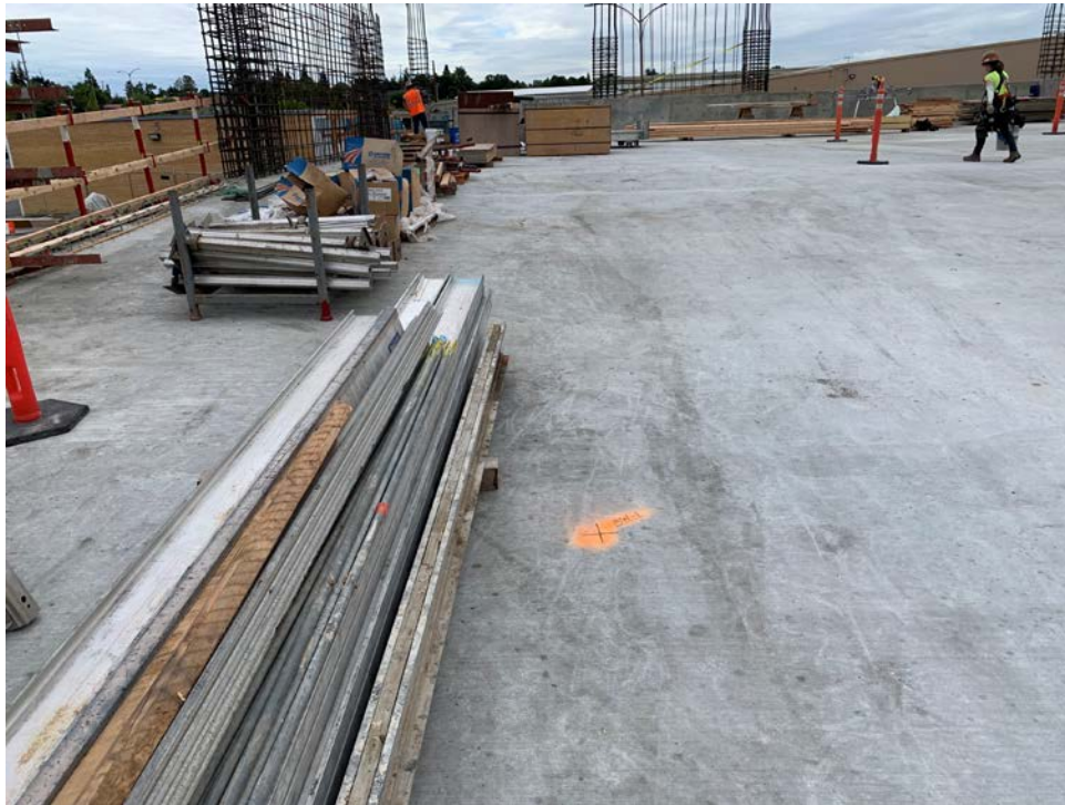
Approximate location of destroyed monitoring well MW-1 within parking garage structure.
