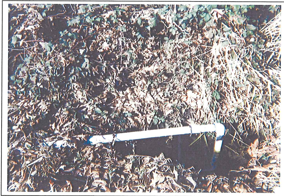
Photo 14. Ditch area along western boundary. The sump near building structure empties into this section of ditch. Pipe observed exiting ditch parallels ditch then runs uphill to West Bay Drive. Discharge point unknown (2/12/04).
