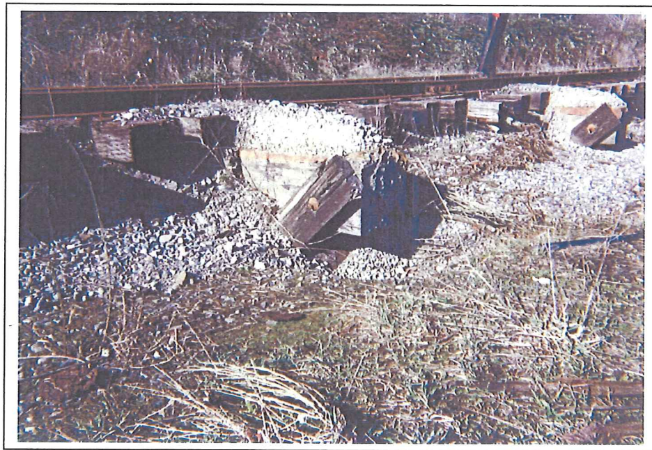
Photo 16. Evidence that rail truss was filled. Center of photograph a rail truss support structure with vertical piling, horizontal metal-capped rail deck beam, with cross member support. A second one observed right corner of photograph, note undisturb rock on rail deck beam and small pile of rocks at the end of beam on the ground. Approximately 18-21 inches of subsidence has occurred on rail spits south of the site (2/12/04).
