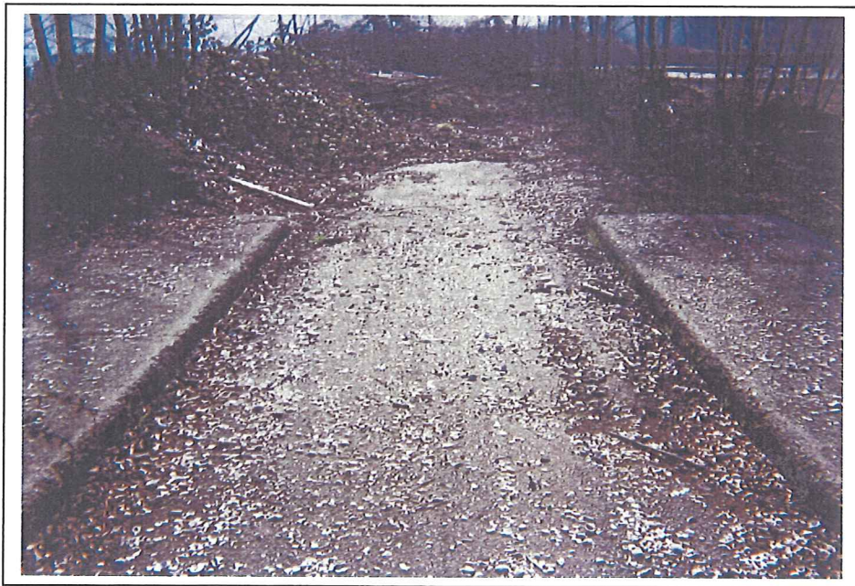
Photo 4. Concrete pad appears to be a containment pad for railroad cars, facing south (2/12/04).
