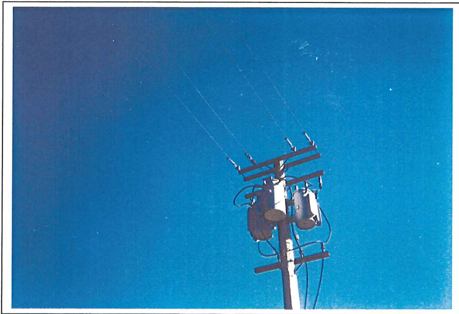
Photo 10. Electrical pole containing transformers (2/12/04).
