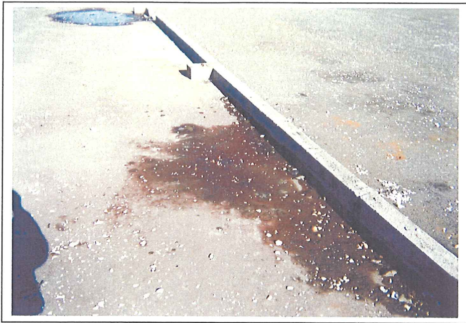
Photo 5. Staining observed within the building foot print, along east wall (2/12/04).
