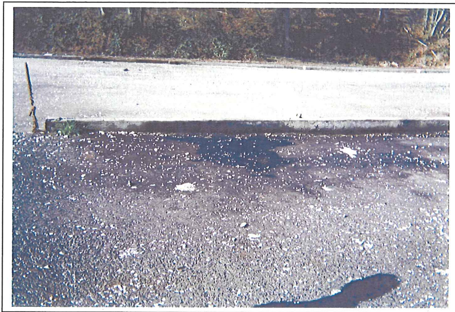
Photo 6. Staining observed exterior of the building along the east wall (2/12/04).
