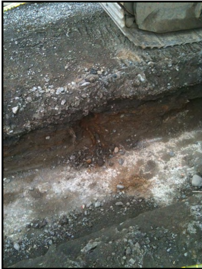
Figure 9. Overview of concrete exposed during utility excavations at the project area, approximately 2 ftbs.
