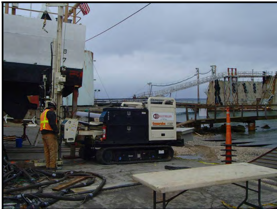
Figure 4. View of Geoprobe®, direct-push technology drill, with shipway rails and WWII-era drydock in background.
