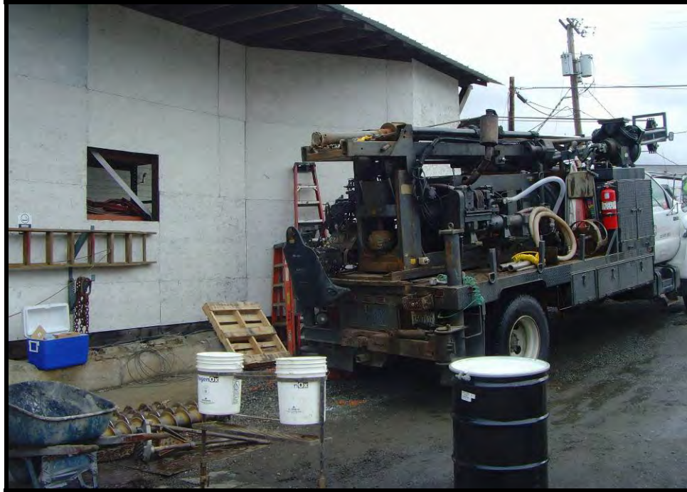
Figure 3. View of truck-mounted auger used to install groundwater monitoring wells at the Harris Avenue Shipyard.
