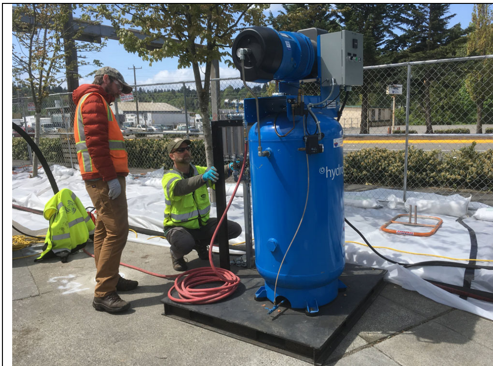
Photo #8: Initiating startup of the AS system, to blow into shallow well AS-1. AS-1 is located beneath the yellow jacket; concerns were raised about pressurizing PVC so a jacket was placed over the well attachment to protect personnel from PVC pieces in the event that the PVC
