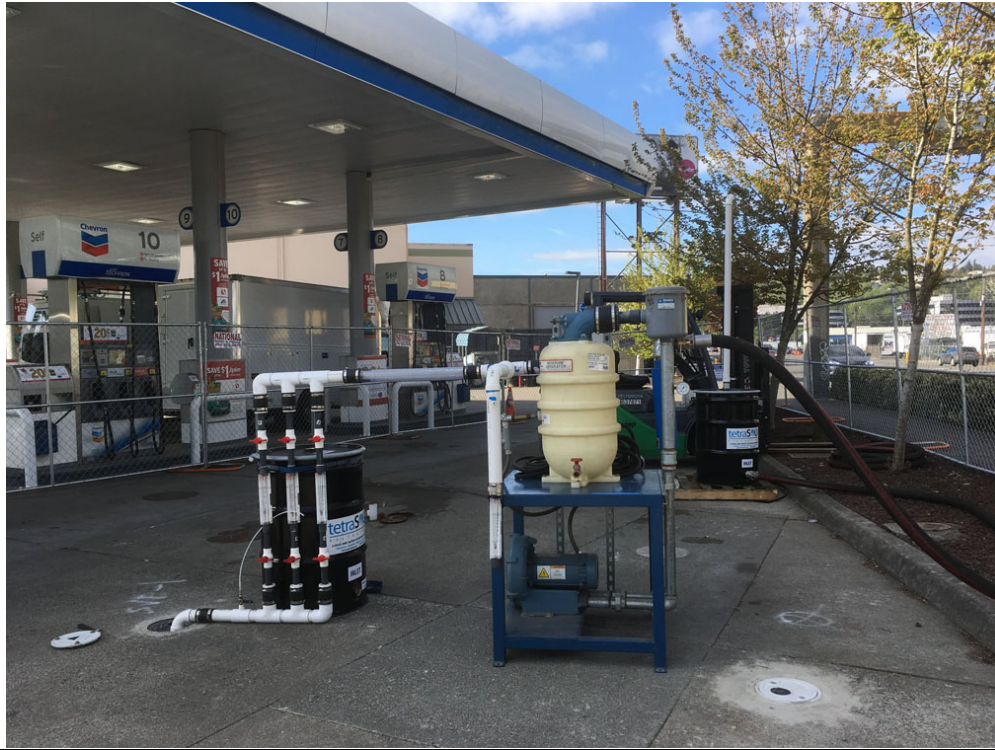
Photo #1: Soil Vapor Extraction (SVE) system set up at well SVE-1. SVE system set up to extract from SVE-1 with manifold with several flow meters in order to conduct a step test. Extracted vapor will be run through GAC canister (drum in background).
