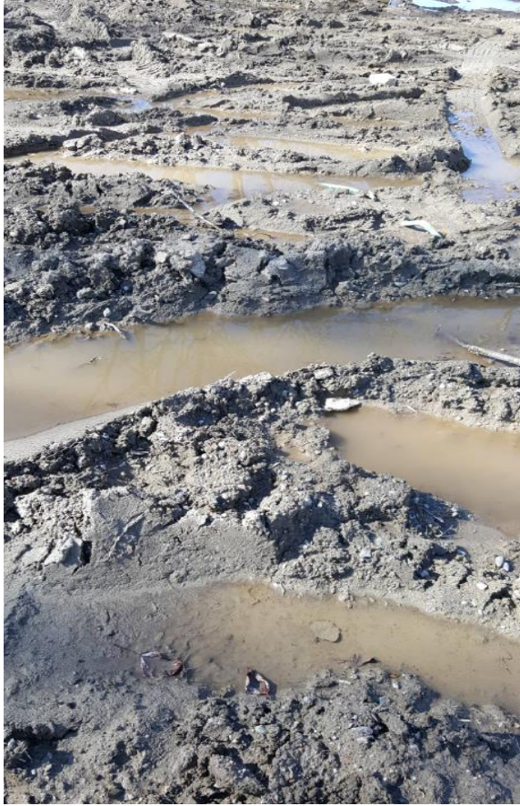
Soil displacement near SS-2
