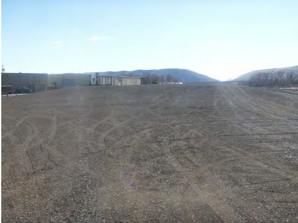
Photograph 17: Northern side of BNSF main cell and BNSF tracks from northern end of cell, looking south.
