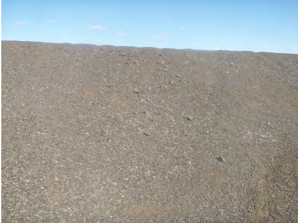
Photograph 11: Quad tracks, burrow, and riprap at southern end of BNSF main cell, looking north.
