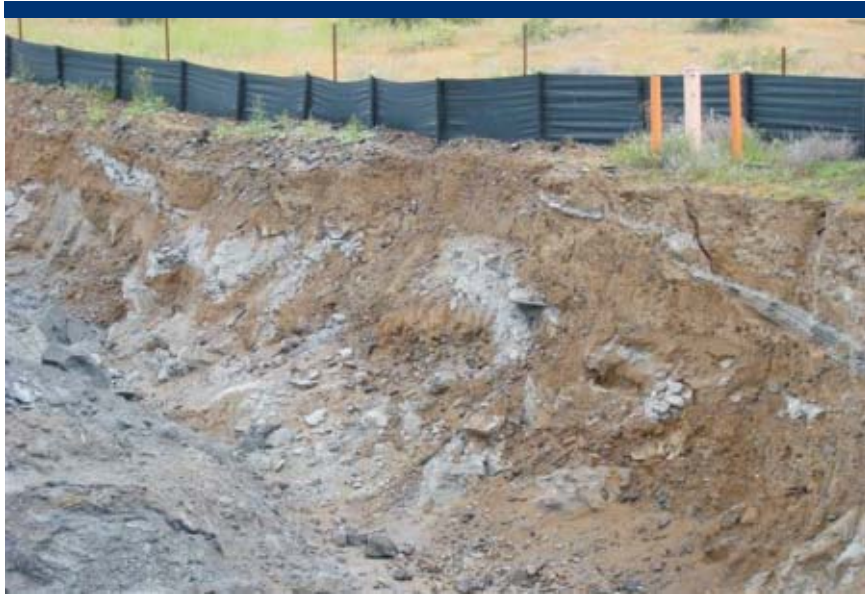
Photo 5 Sidewall and dross embedded in matrix. Monitoring well MW-3. Silt fence is Army Corps property line. Direction: Northeast Date: 5/6/09
