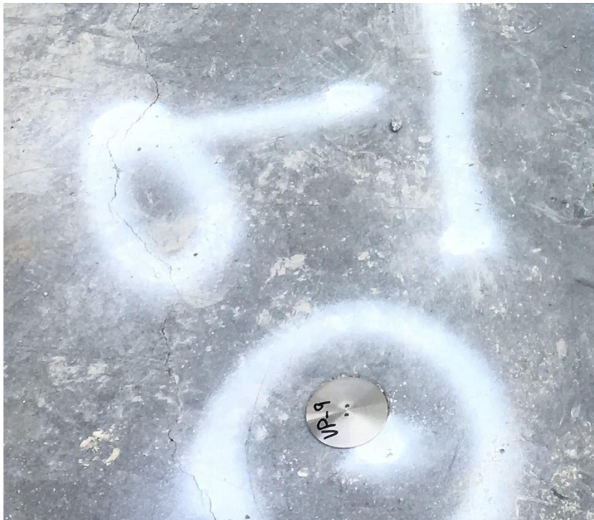
Photograph 4. Vapor pin with flushed-cover.
