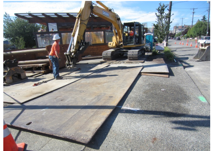
Photograph 4. Covering an open excavation with steel plates at the end of the day.
