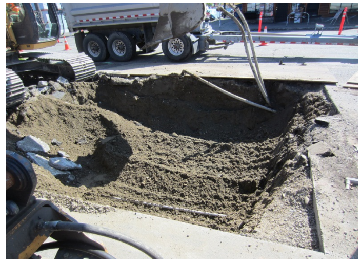
Photograph 2. Exposed abandoned pipes.
