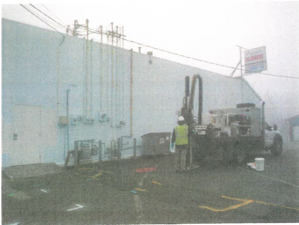
Figure 10. Location of Boring 2. Door in left side of photo is back door to the dry cleaner, currently utilized by Olympic Cleaners.
