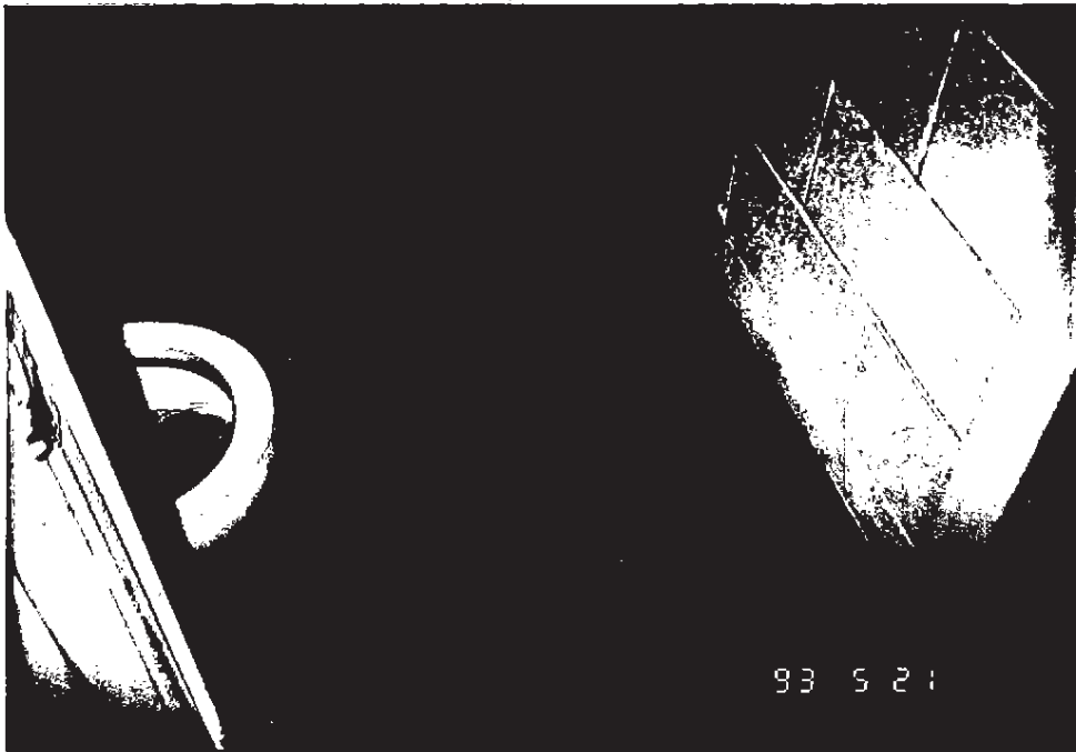
Photograph 19 Floor tile, which is a suspect ACM.
